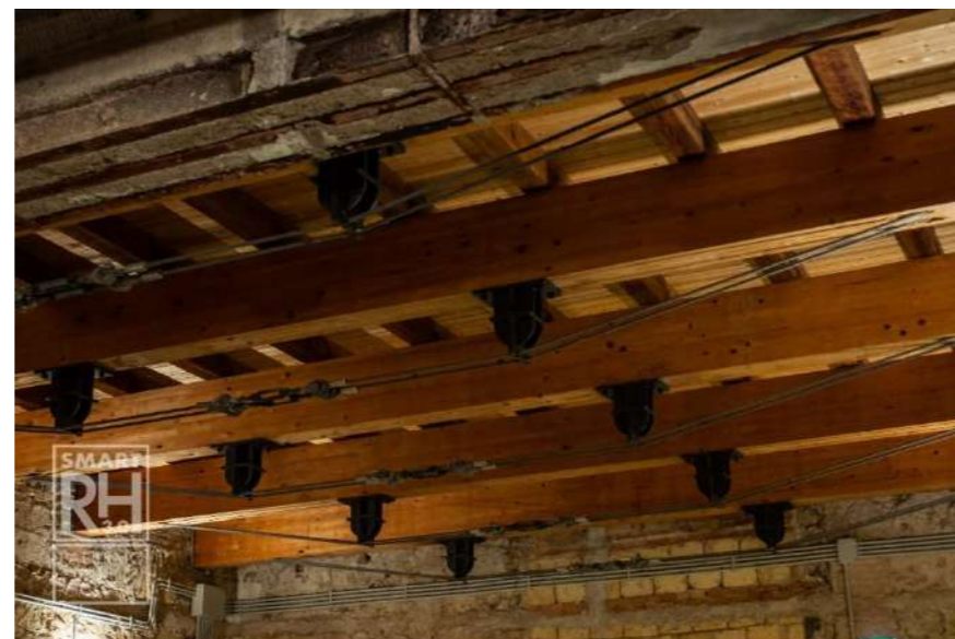
Fig.9b: New wooden floors; detail of the reinforced wooden beams. © Francesco Renda
