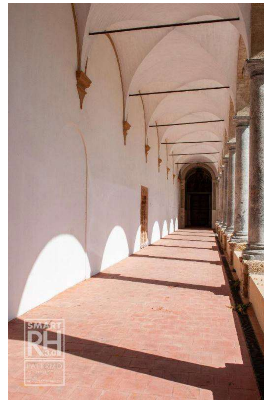
Fig.6b: Detail view of one of the arms of the inner portico with stone cross vaults, set on corbels and metal chains to eliminate horizontal actions. ©Francesco Renda
