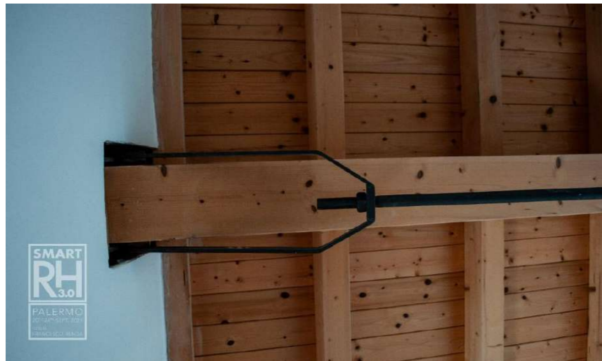
Fig.11a-b: View of new timber structure of a roof with steel tie rods to eliminate pushing actions. ©Francesco Renda
