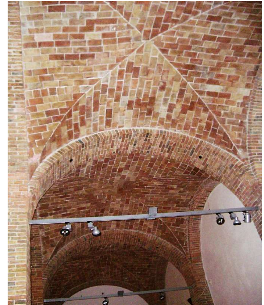
Fig.22: The new timbered vaults, after reconstruction works. © Municipality of Palermo, Historical Center Technical Area
