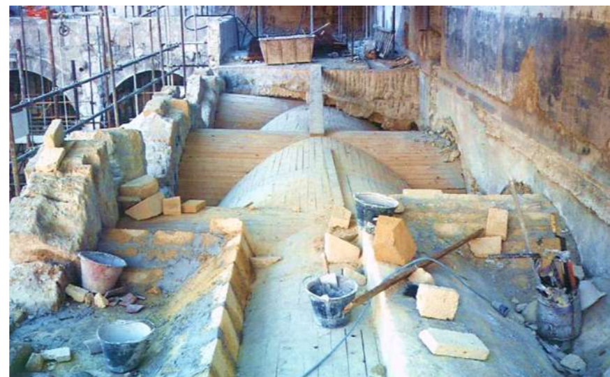
Fig.21: Collapse of an arm of the porch of the convent, following a mafia attack and start of the reconstruction and restoration works: reconstruction of stony vaults. © Municipality of Palermo, Historical Center Technical Area
