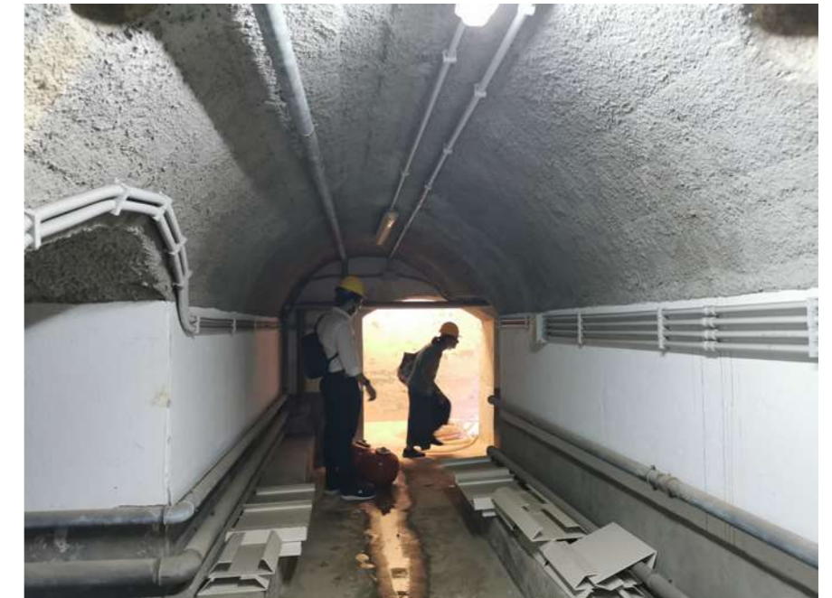
Fig.31: Air-raid shelter below the courtyard of the convent, now used to house the integrated services. © Luisa Lombardo
