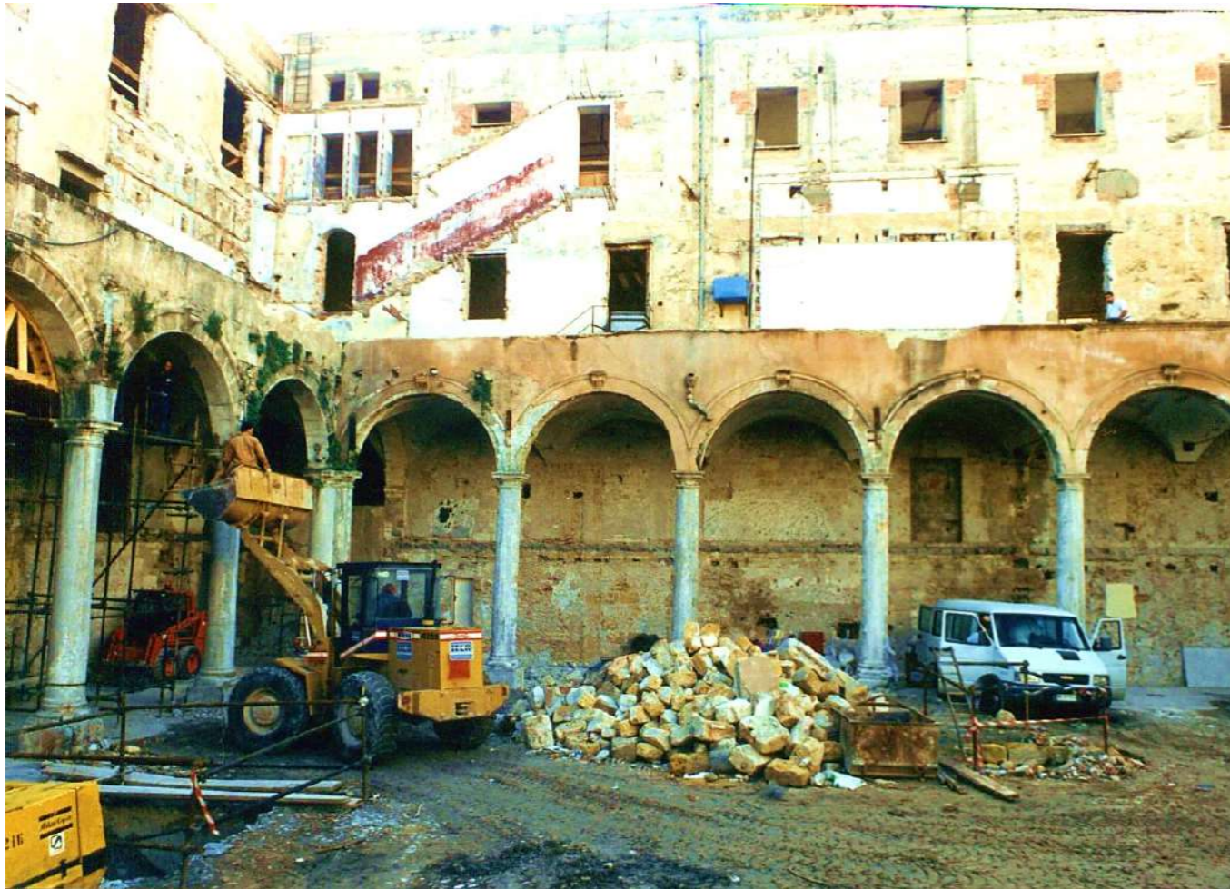
Fig.9: Start of demolition and restoration work on the convent portico. © Municipality of Palermo, Historical Center Technical Area
