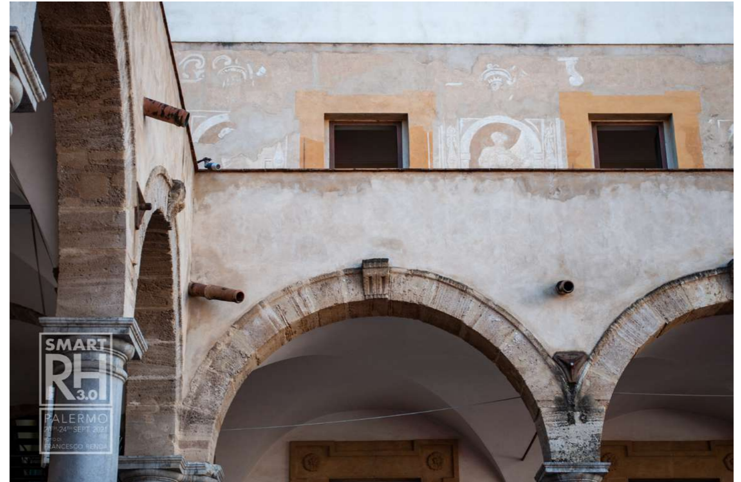
Fig.10: Detail of the arcades of the portico, after the restorations. © Francesco Renda
