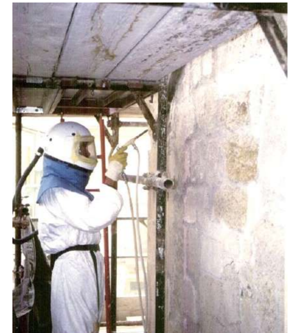
Fig.13: Micro-aero-abrasive cleaning interventions of the shell limestone wall faces. © Municipality of Palermo, Historical Center Technical Area
