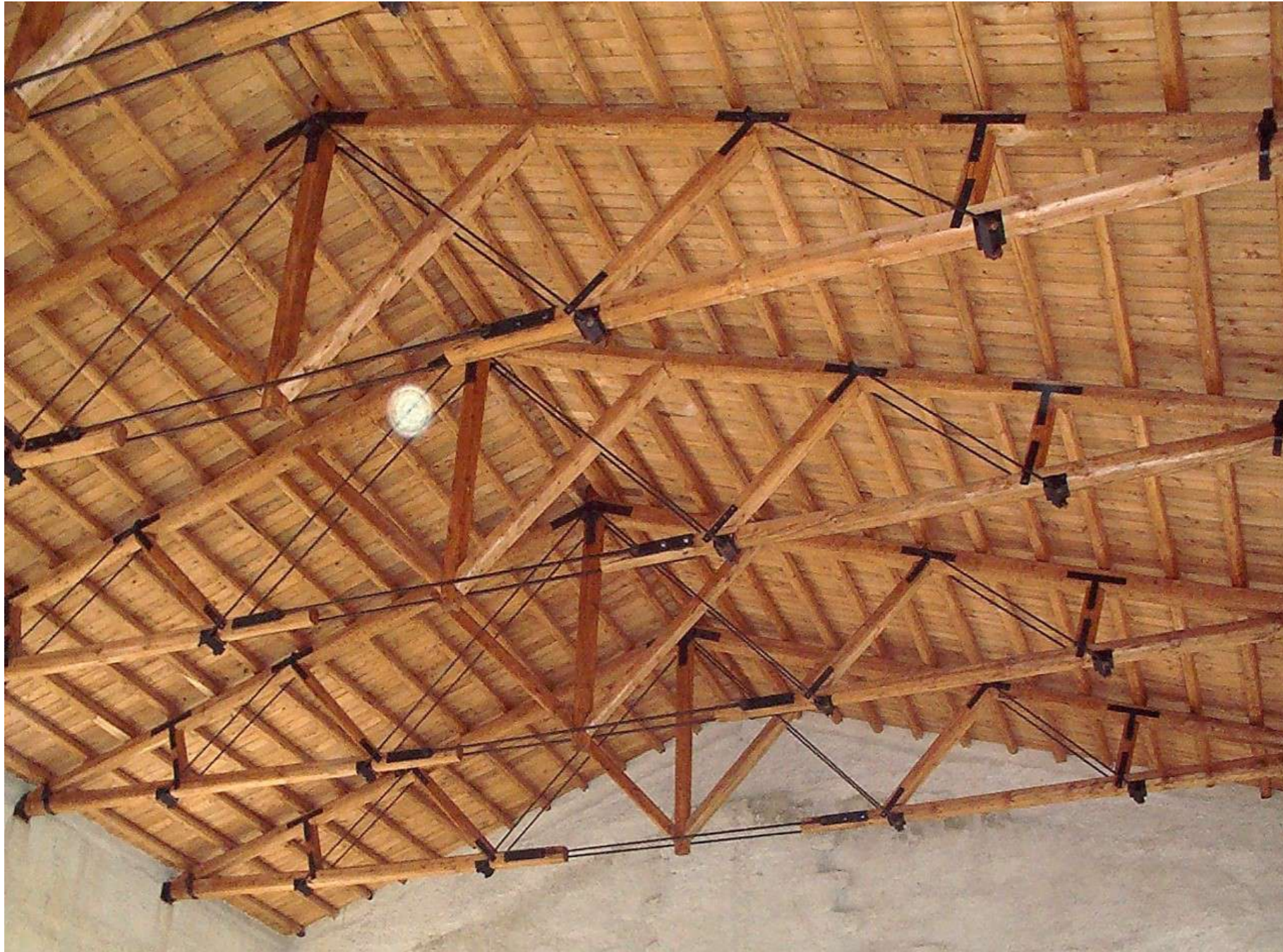
Fig.28: Consolidation works and structural reinforcements on wooden roofs. © Municipality of Palermo, Historical Center Technical Area
