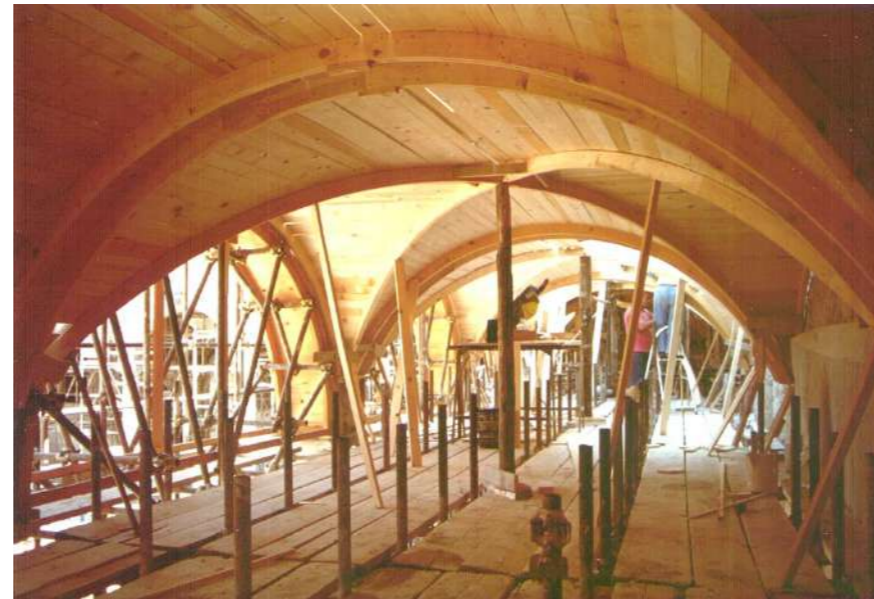
Fig.20a-b: Collapse of an arm of the porch of the convent, following a mafia attack and start of the reconstruction and restoration works: wooden centering useful for the reconstruction of stony arches and vaults. © Municipality of Palermo, Historical Center Technical Area
