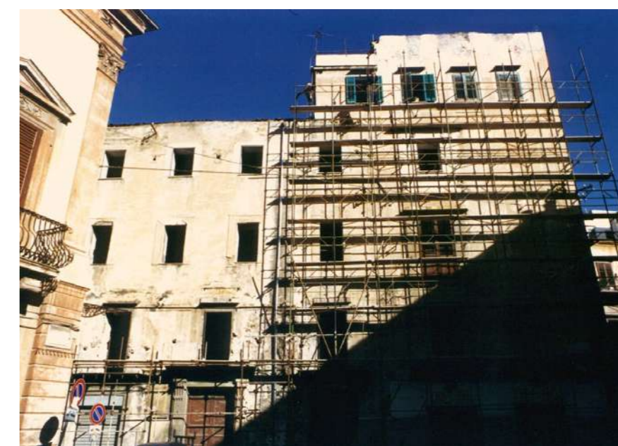
Fig.2: The façade along the Croce dei Vespri square, during the restorations. © Municipality of Palermo, Historical Center Technical Area
