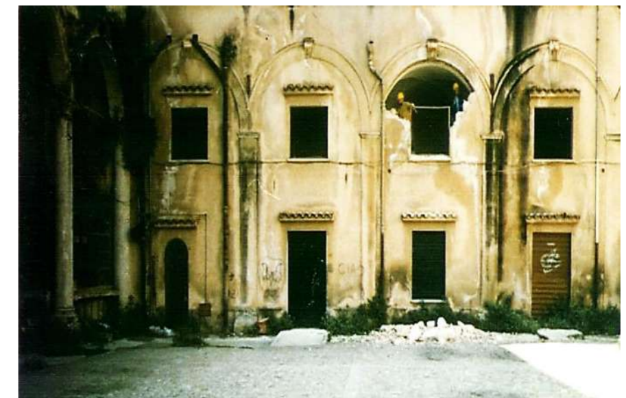
Fig.8: The arches of an arm of the convent portico, before the restoration, with the stony arches closed by incongruous masonry. © Municipality of Palermo, Historical Center Technical Area
