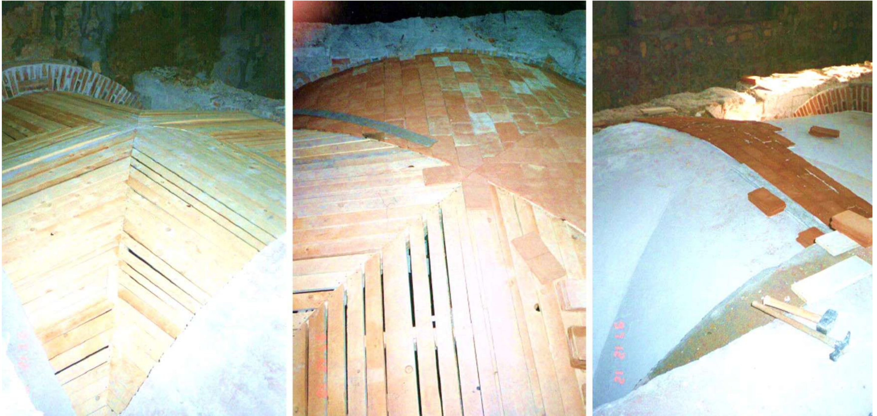
Fig.23: Reconstruction of collapsed brick timbered vaults. © Municipality of Palermo, Historical Center Technical Area
