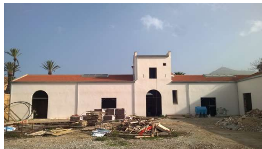
Fig.11: East façade facing the internal courtyard after reinforcement and cleaning. © Arch.Chiara Mazzarella
