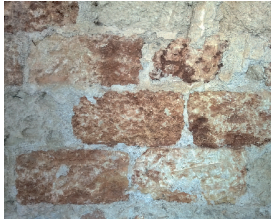
Fig.24b: The Vinery during the construction phase; detail of the existing masonry. © Arch.Chiara Mazzarella
