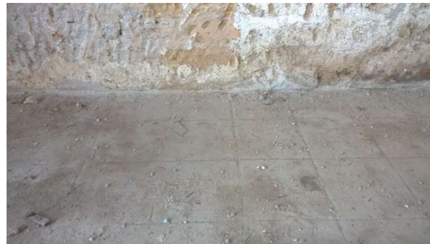
Fig.25: The winery. Floor detail before the rehabilitation. © Arch.Chiara Mazzarella
