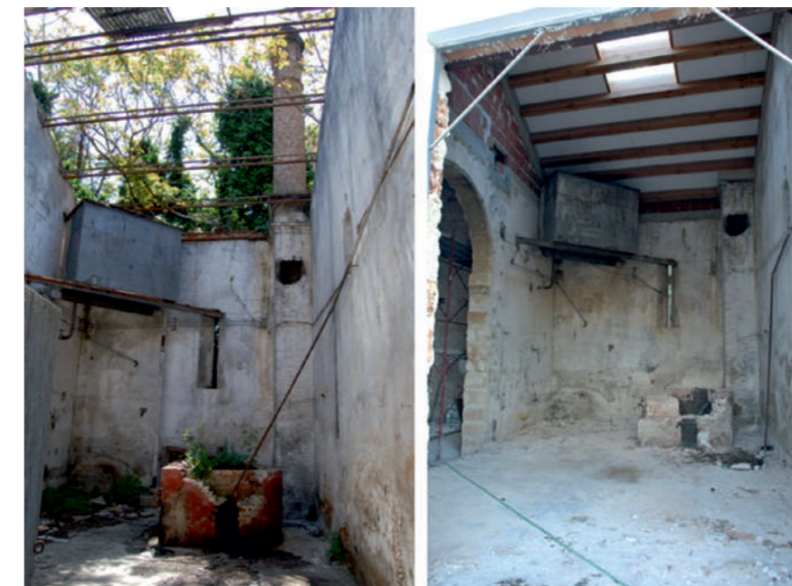
Fig.12: Delicatessen space before and after in the construction site. Original chimney and tanks were maintained. © Arch.Chiara Mazzarella
