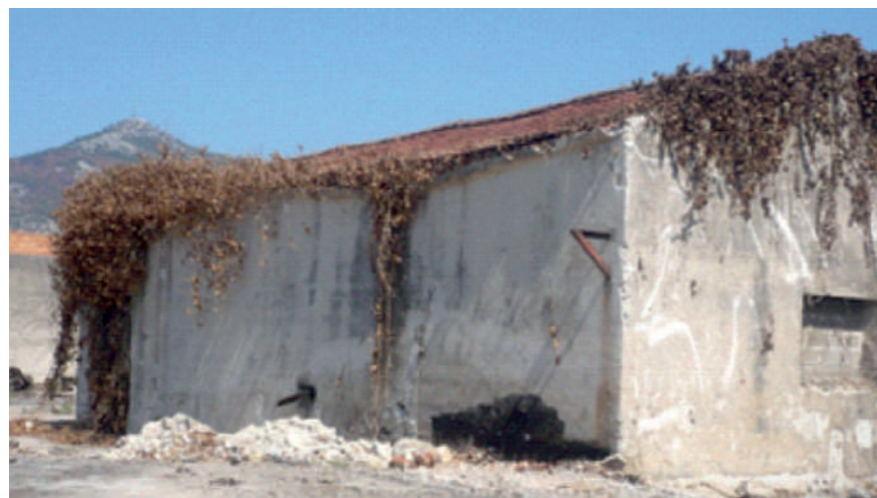
Fig.8a-b: Façades on the internal court before the rehabilitation. © Arch.Chiara Mazzarella
