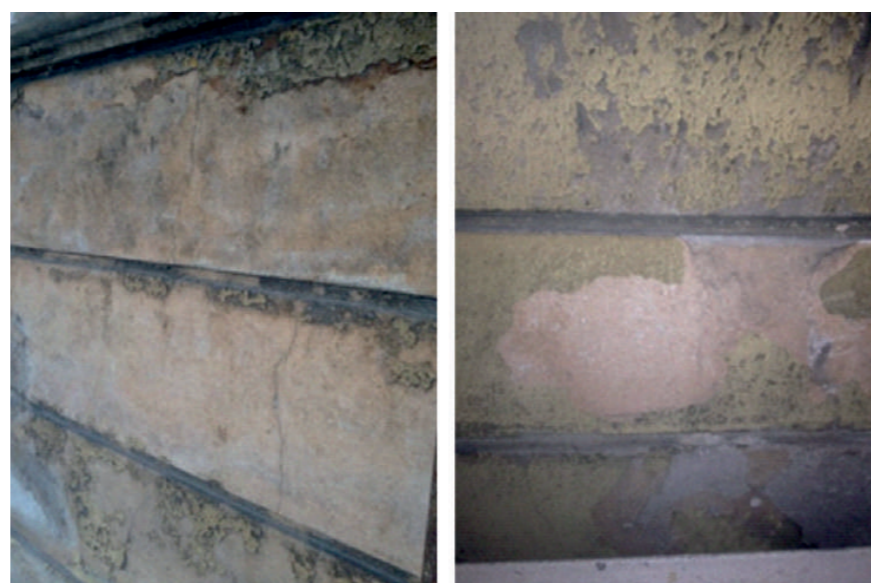
Fig.6: Nord façade along San Lorenzo Street and focus on the original plaster before the rehabilitation. © Arch.Chiera Mazzarella
