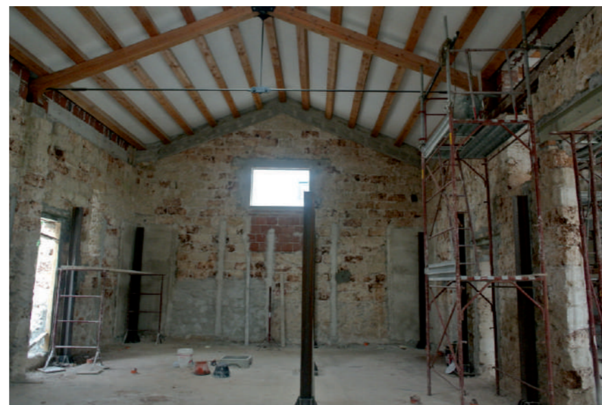
Fig.18: Ice-cream shop, during the construction phase; Construction of iron lofts. © Arch.Chiara Mazzarella
