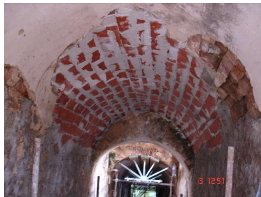
Fig.9: State of maintenance of a brick-made vault, with partial structural failure and diffuse degradation. @ Eng. Marinella Fiore
