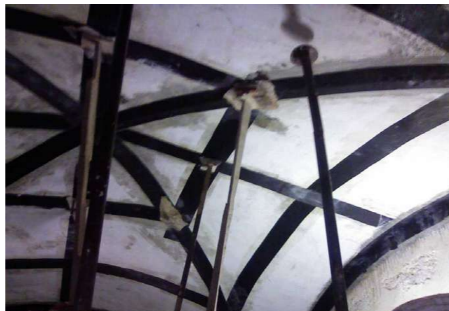
Fig.16: Reconstruction of stone vaults with carbon fibres reinforcement (FRP), view of the intrados. @ Eng. Marinella Fiore
