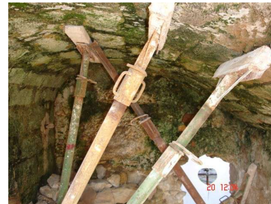
Fig.10: A propped-up vault to avoid further collapses waiting for the restoration work. @ Eng. Marinella Fiore
