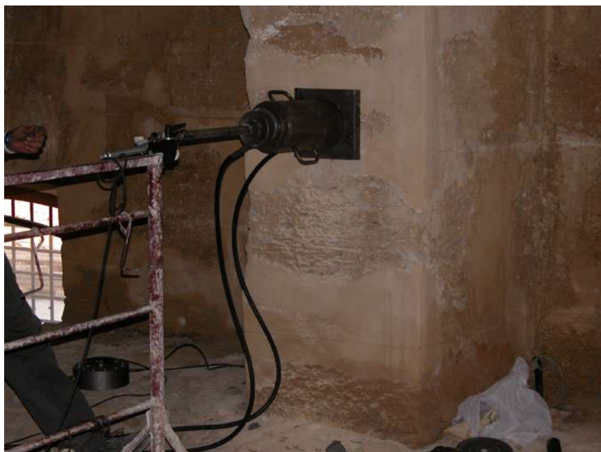
Fig.14: Restoration of the load-bearing masonry and verification of its structural integrity, during the restoration works. @ Eng. Marinella Fiore
