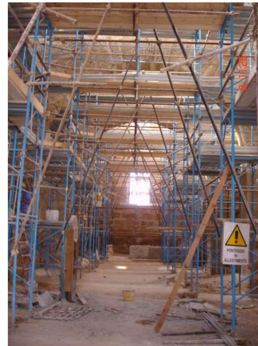
Fig.13: The inner nave with the scaffold, during the restoration works. @ Eng. Marinella Fiore
