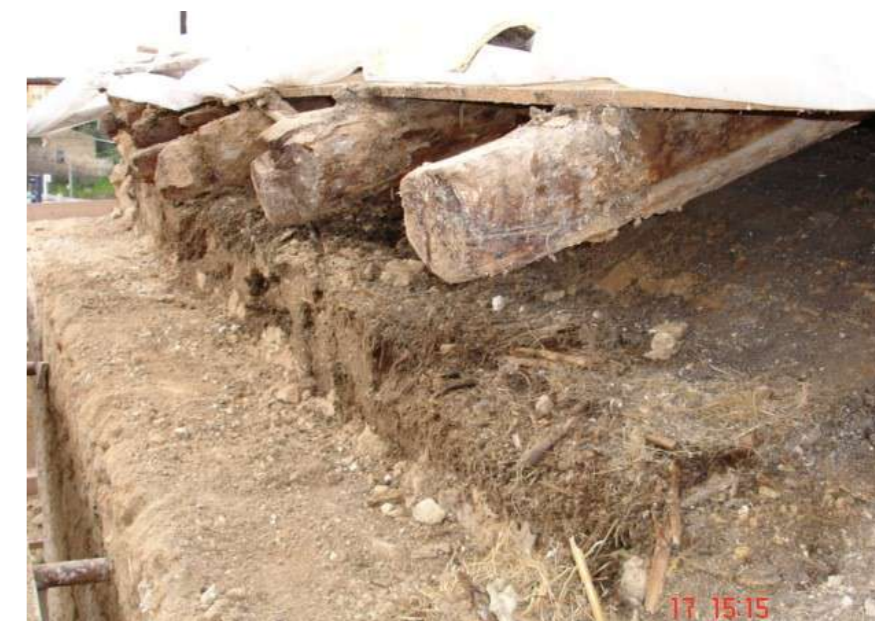
Fig.11: State of maintenance of the wooden roofs, with diffuse collapses, lack of material, degradation of the heads of the beams, bird nests and vegetation. @ Eng. Marinella Fiore
