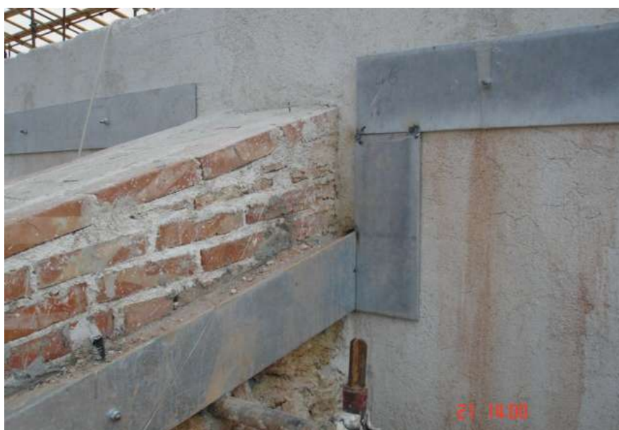
Fig.15: Construction of curbs, made of reinforced concrete, located at the walls' top to ensure a box-like behavior and avoid future collapse, during the restoration works. @ Eng. Marinella Fiore
