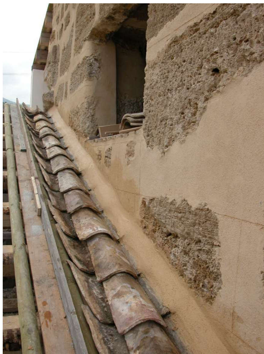
Fig.20: Reconstruction of the roofs, installation of traditional terracotta tiles (Sicilian coppo), during the restoration works. @ Eng. Marinella Fiore
