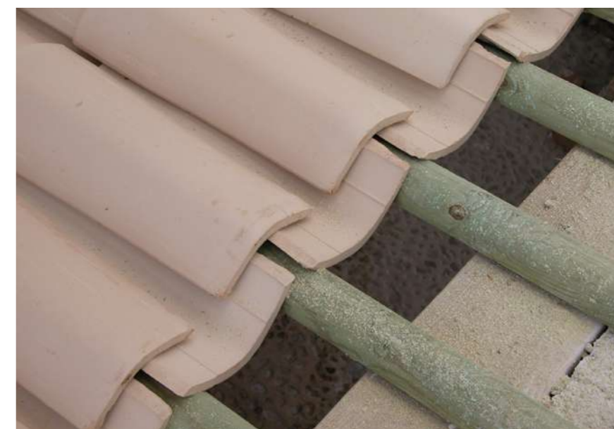
Fig.19: Reconstruction of the roofs, installation of half smaller wooden beams on the main wooden ones, surmounted by corrugated plank, during the restoration works. @ Eng. Marinella Fiore
