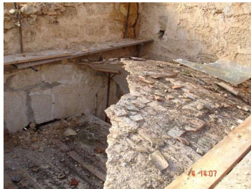
Fig.8: State of maintenance of the vaults, with diffuse collapses. @ Eng. Marinella Fiore
