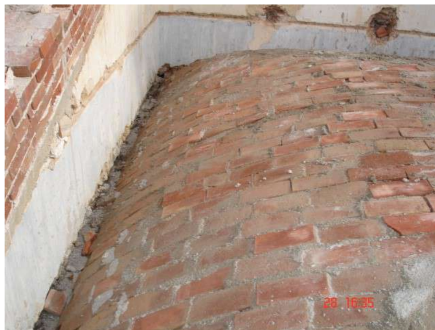
Fig.17: Reconstruction of stone vaults, view of the just finished extrados, during the restoration works. @ Eng. Marinella Fiore
