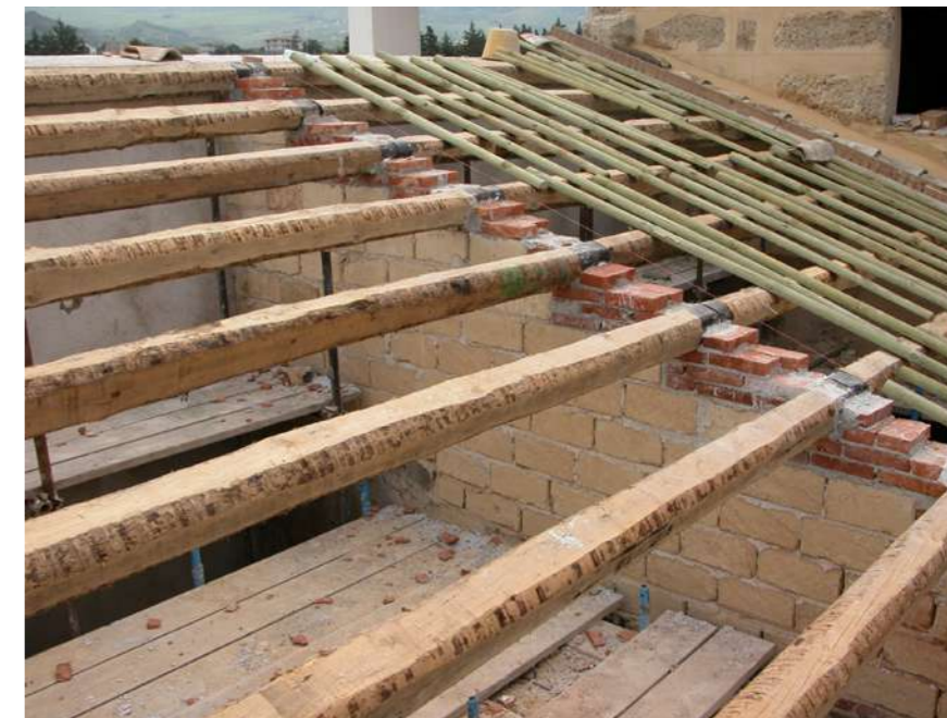
Fig.18: Reconstruction of the roofs through the installation of main wooden beams, surmounted by half smaller wooden beams, during the restoration works. @ Eng. Marinella Fiore
