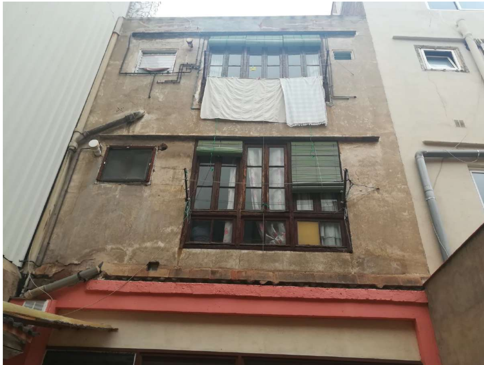
Fig.14: Previous state of the courtyard's façade.
