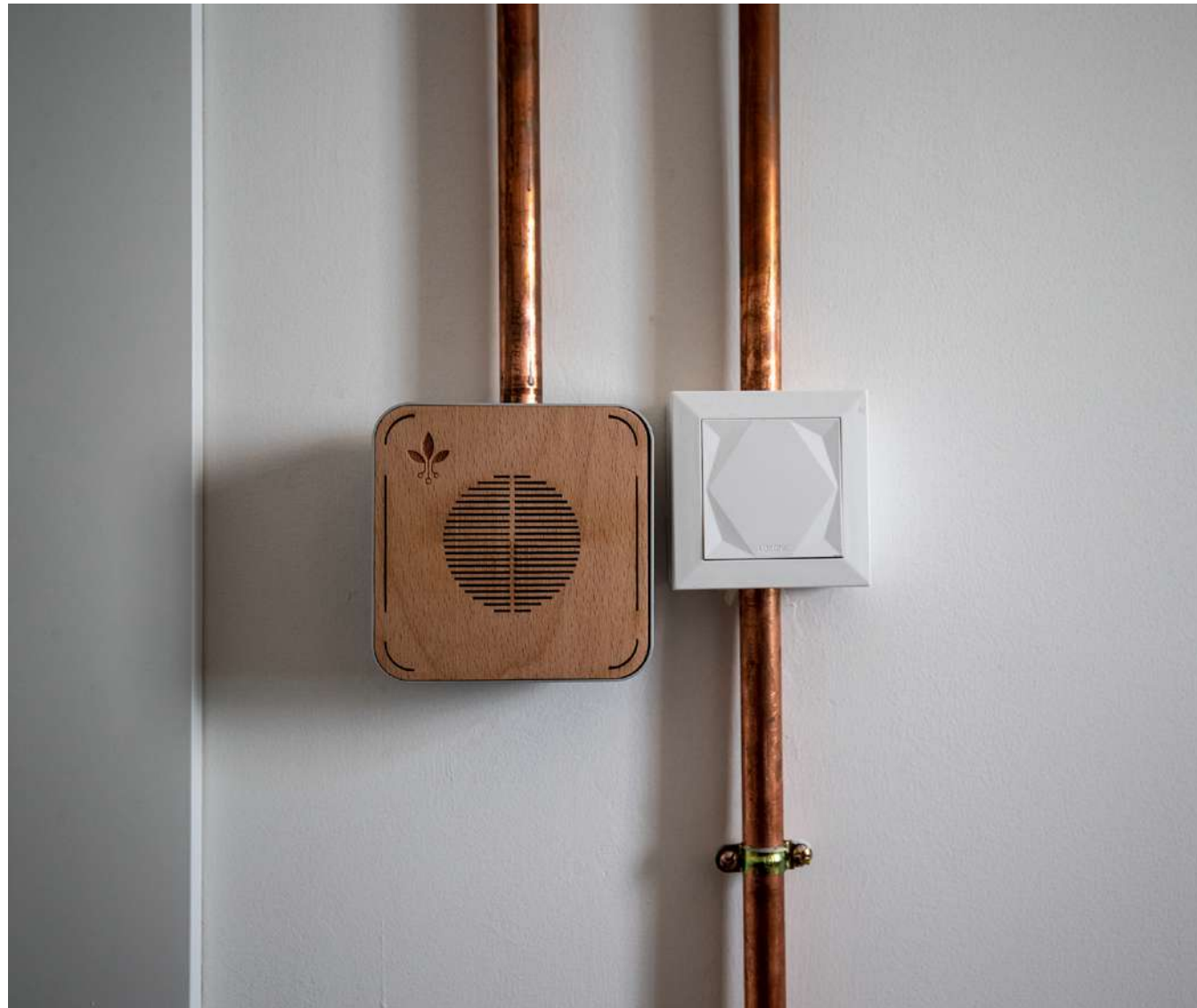
Fig.18: Monitoring and improvement of indoor air quality.
