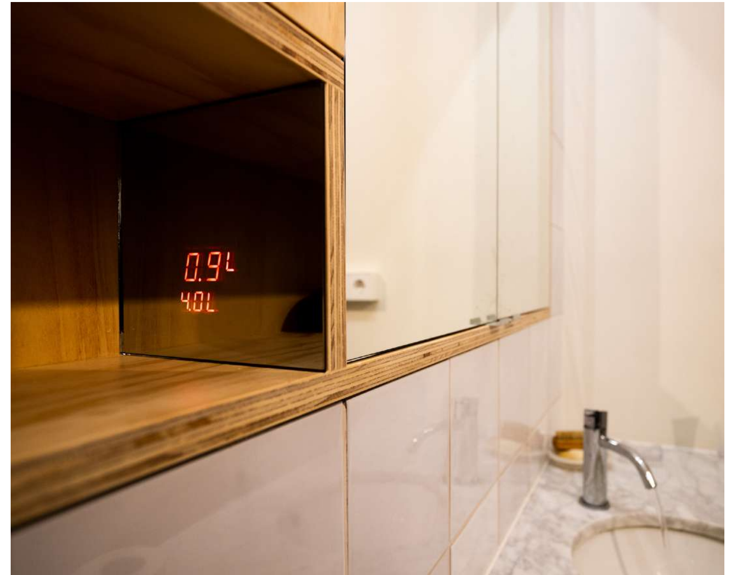
Fig.19: Hot water consumption meter.
