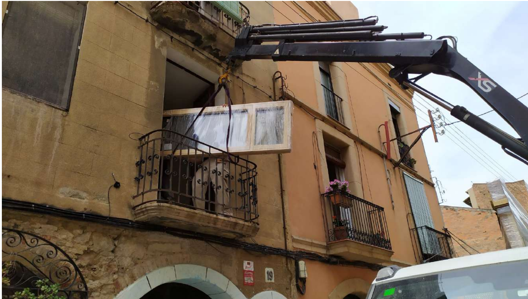
Fig.12: View of the intervention works, transporting the new windows, and the existing conditions of the main façade can be seen on this image.
