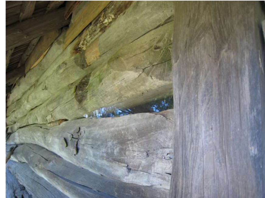
Fig.11: Rent cracks filled with glass.
