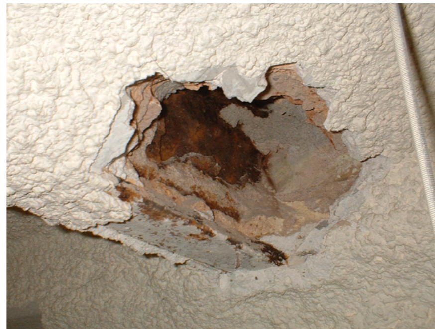
Fig.2: Heads of rusty-exfoliated profiles in support area (inside the masonry wall and lime mortar).
