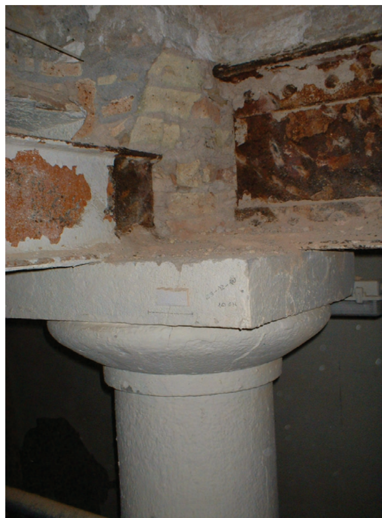
Fig.10: Existing conditions prior to the rehabilitation of the capitel and head of the composite profile beam.
