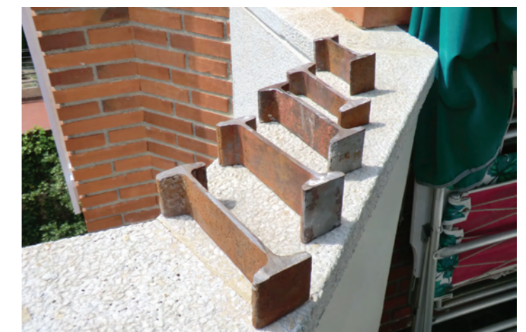
Fig.3-4: Rusted and swollen profiles; Fig.5: Narrow-wing profiles used in the building.
