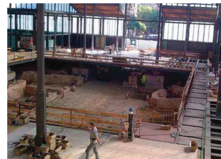
Fig.3: View of the execution of the new floor slabs, and the archeological excavations underneath.
