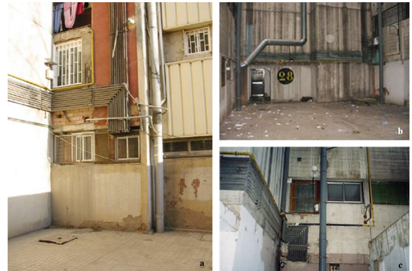
Fig.7: Condition of the facilities prior to the intervention.
