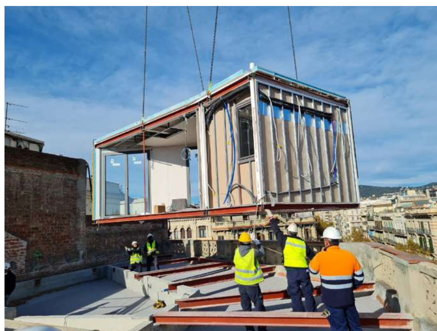
Fig.6: Installing the pre-fabricated modules on its final resting place on the roof.
