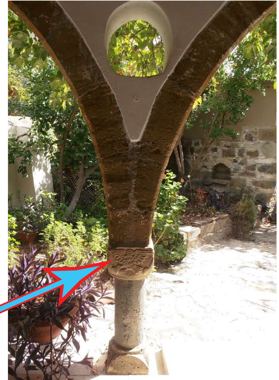
Fig.9-10: The main column supporting the arches of the portico had its deteriorating capital replaced while a second capital discovered during excavations for its foundation was used as a base. © N. Chrysochou
