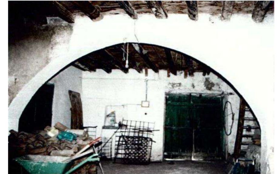
Fig.7-8: Views of the exterior and interior of the dwelling before restoration showing the condition of its structure. © M. Philokyprou
