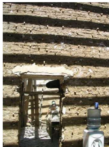
Fig.8-10: Left to right: Revealing the painted ornamentation of the arch of the double room 'dihoron'. Revealing the walls and the roof structures. Adobe work and reinforcement of the wall with wood to receive plater work. © Y. Hadjichristou
