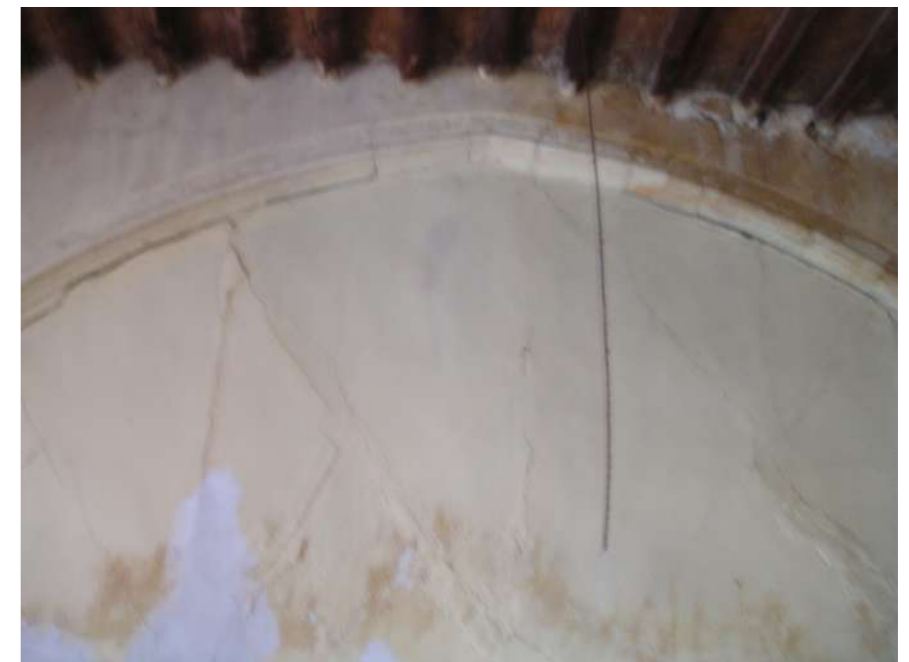
Fig.5-6: Falling walls due to leakages and abandoness. The arch of the double room 'dihoron' with hidden painted ornaments. © Y. Hadjichristou
