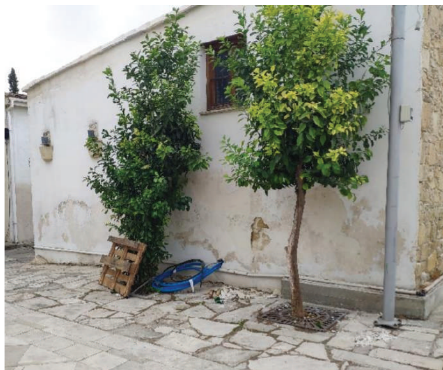
Fig.4: View of the building before restoration. © FOSS Research Centre for Sustainable Energy / University of Cyprus
