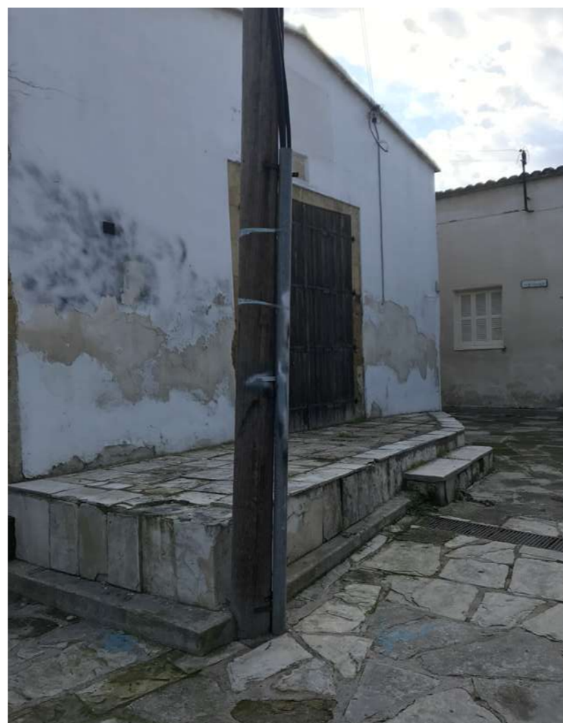
Fig.5: View of the building before restoration. © FOSS Research Centre for Sustainable Energy / University of Cyprus
