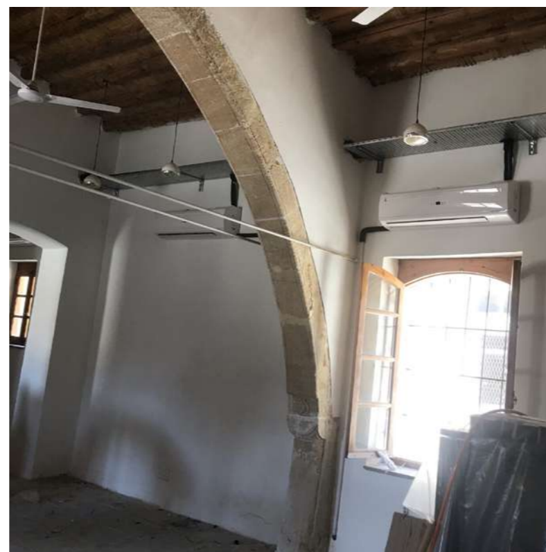
Fig.26: HYBUILD System installation. © FOSS Research Centre for Sustainable Energy / University of Cyprus
