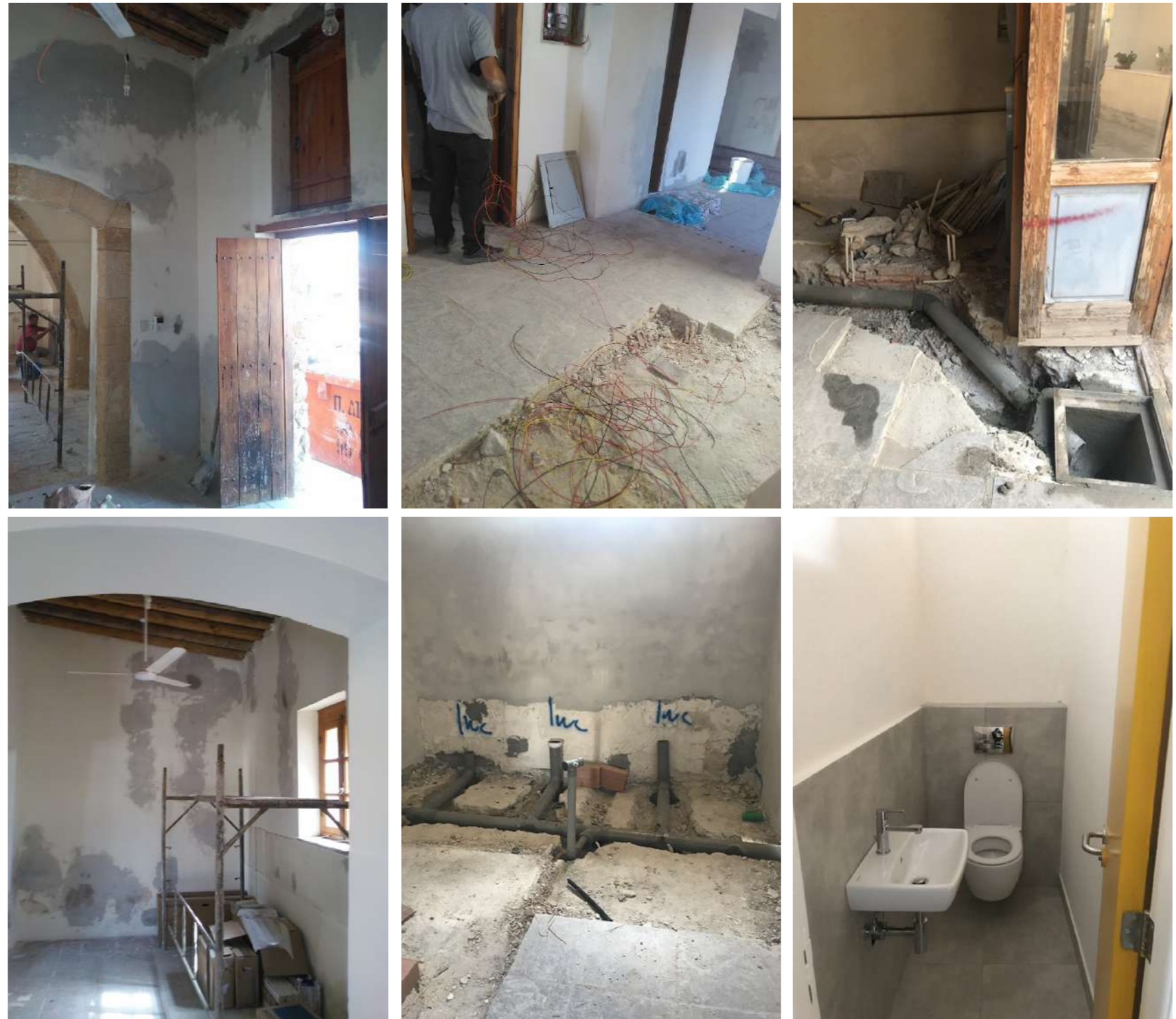
Fig.12-17: Views of the building during conservation. © FOSS Research Centre for Sustainable Energy / University of Cyprus
