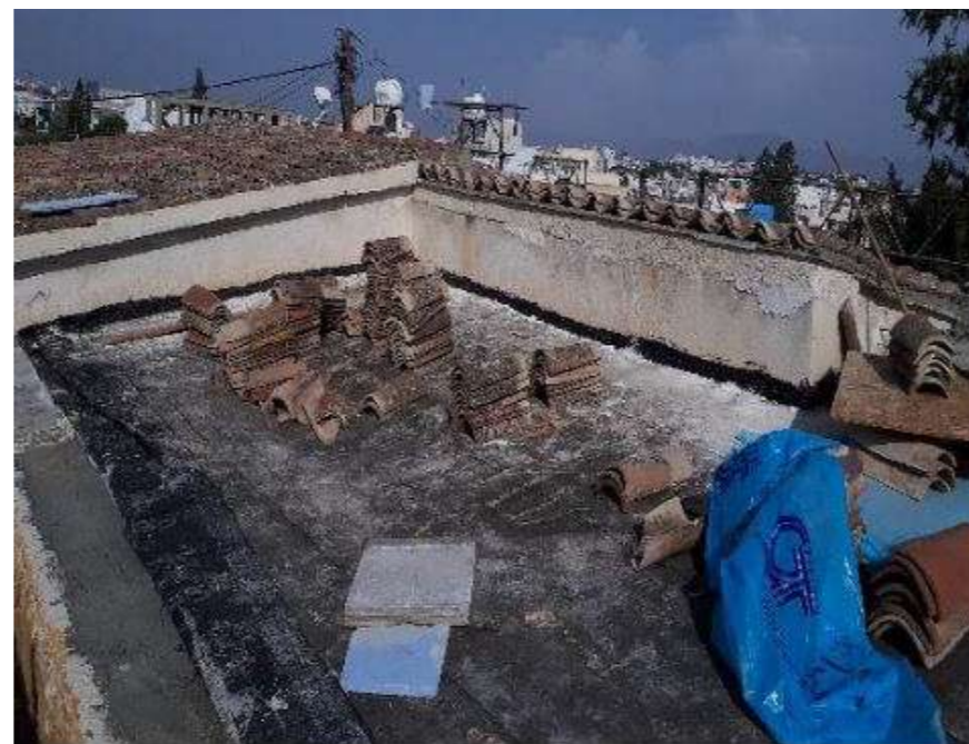
Fig.20-22: Improvement of the roof's thermal performance. © FOSS Research Centre for Sustainable Energy / University of Cyprus
