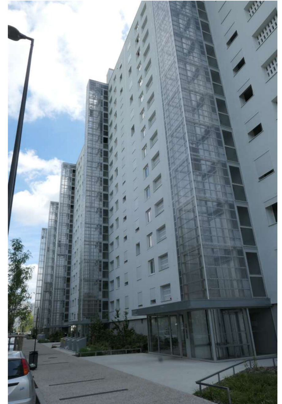
Fig.25: View of the Backside façade of the buildings H & I, with the new rehabilitated staircases and entrances.
