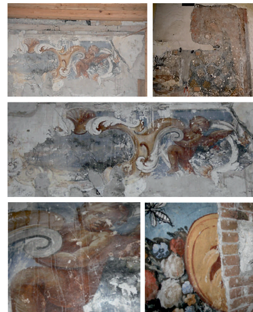
Fig.24: Painted wall surfaces, before restoration. © Arch. Francesco Miceli
