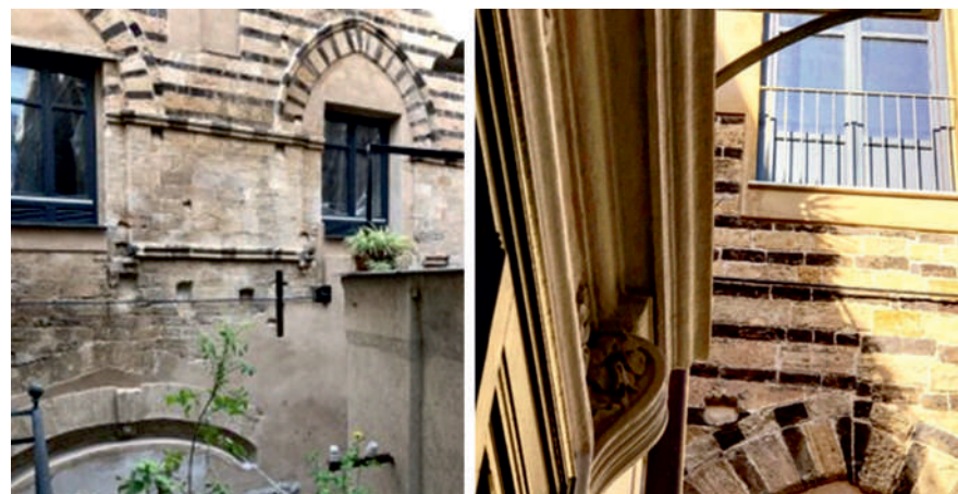
Fig.12: Celso Street's façade. Arches and masonry's details of the planking. © Arch. Francesco Miceli
