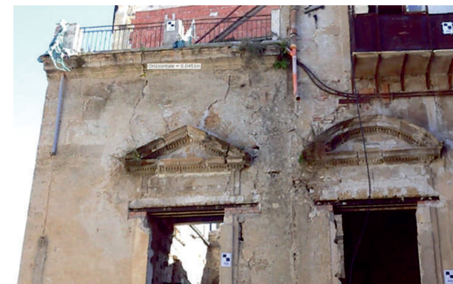
Fig.11: Façades of the inner court. Evident cracks in the upper part before the interventions. © Arch. Francesco Miceli
