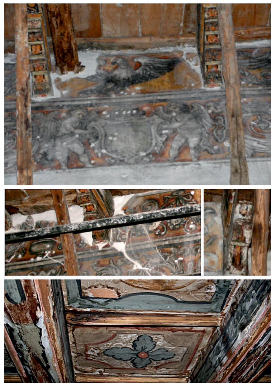
Fig.23: Shelves, beams and wooden coffers inlaid and decorated with paintings before restoration. © Arch. Francesco Miceli
