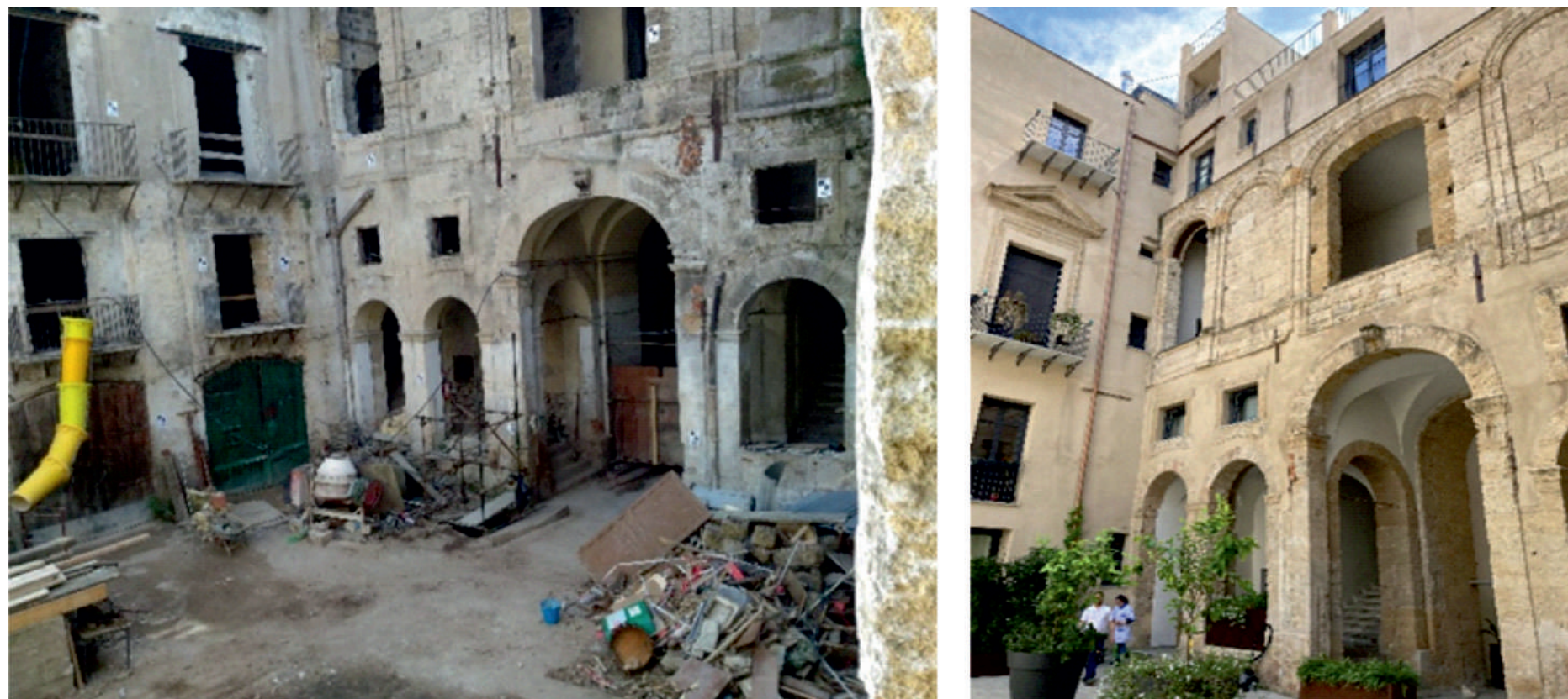
Fig.19: View of the internal courtyard, during the restoring phase and after the restoration. © Arch. Francesco Miceli
