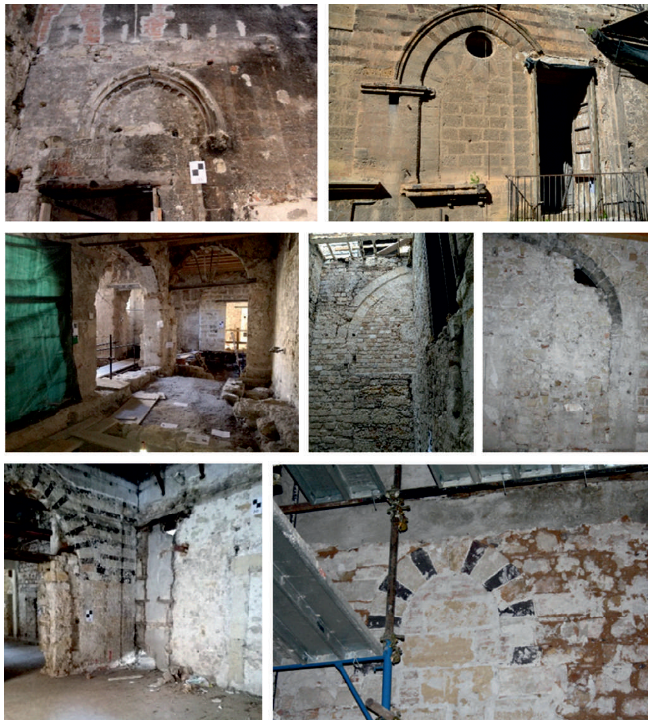
Fig.21: Arches' examples originally present on the elevations, then incorporated into the masonry at different levels. © Arch. Francesco Miceli
