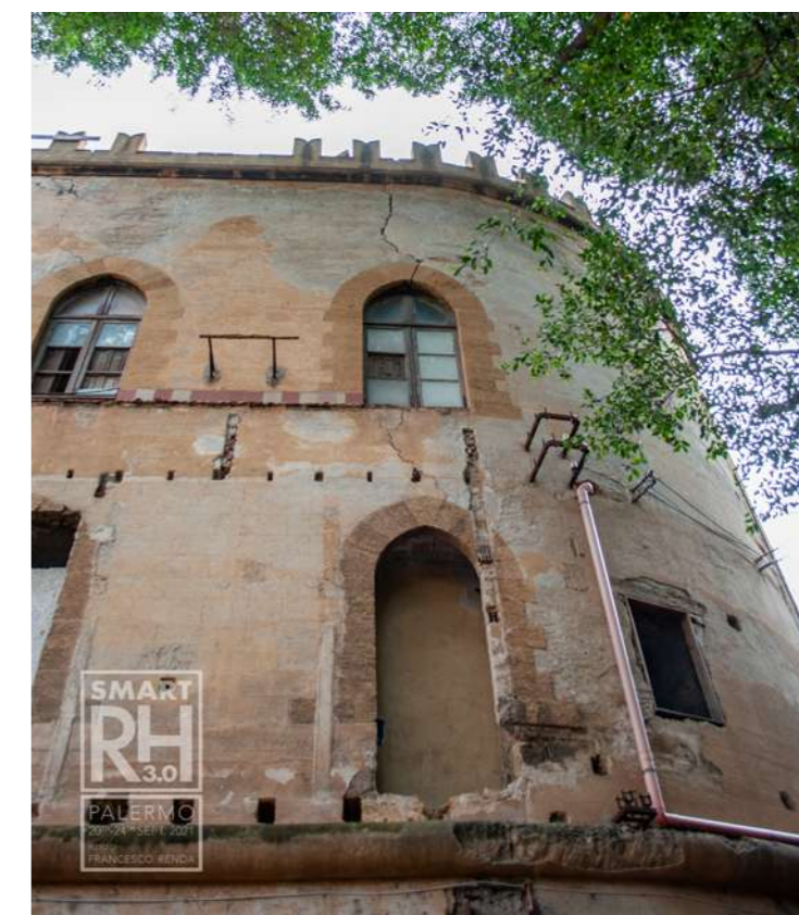
Fig.22: Detail of cracks in the façade of palace tower. © Francesco Renda
