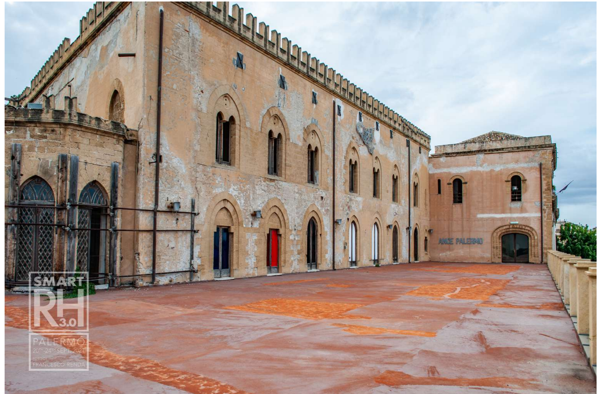
Fig.24: Detail of façade along the waterfront (first floor and terrace): material-construction decay. © Francesco Renda
