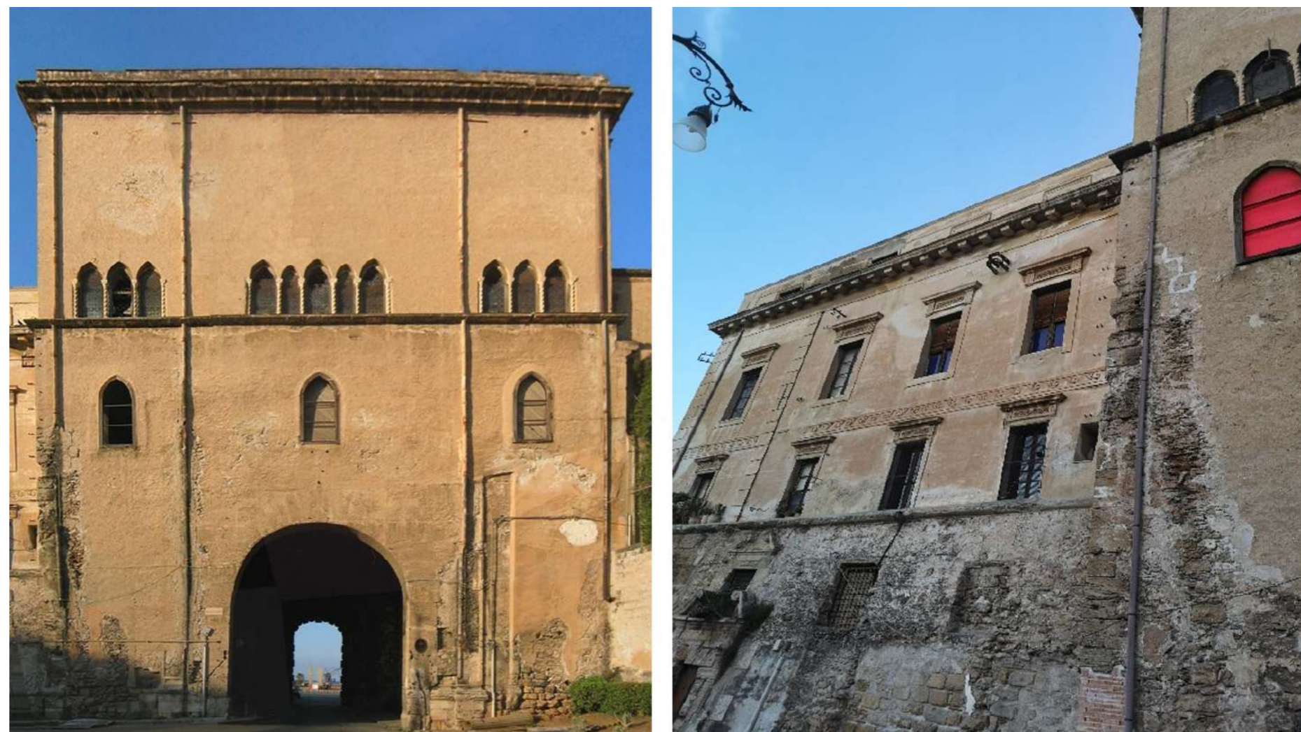
Fig.19a: Façade along Kalsa square: material-construction decay. © Project Designers
