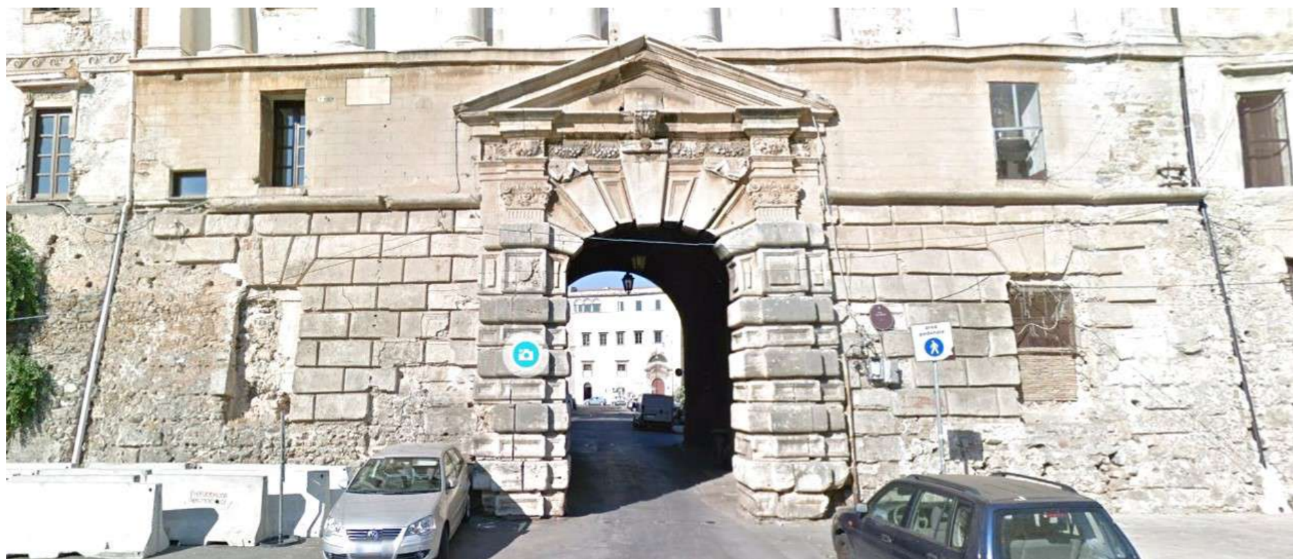
Fig.21: Detail of Façade along the waterfront: material-construction decay. © Francesco Renda
