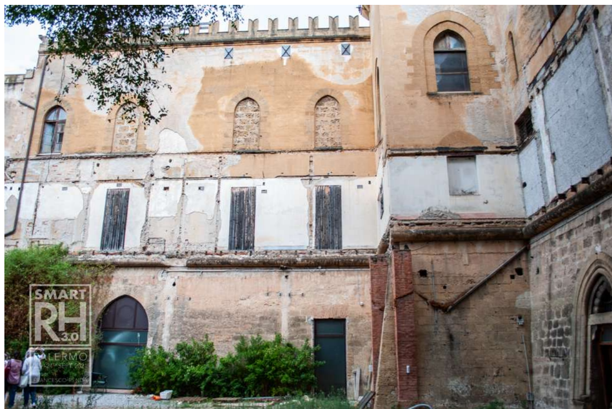
Fig.19d: Façade facing the inner garden: material-construction decay. © Francesco Renda
