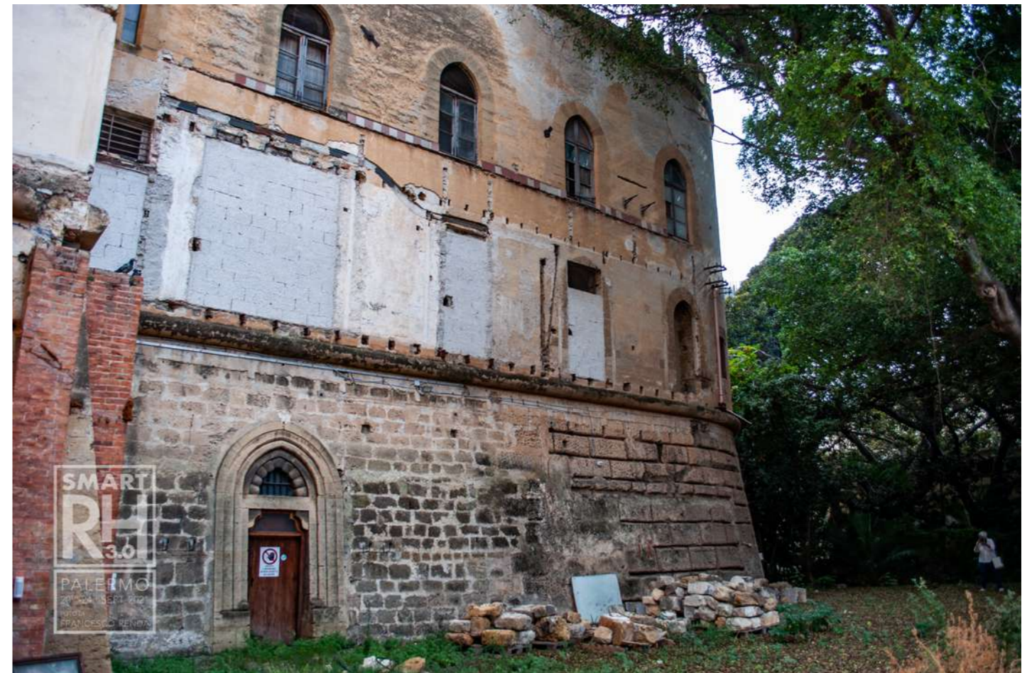
Fig.19c: Façade facing the inner garden: material-construction decay. © Francesco Renda
