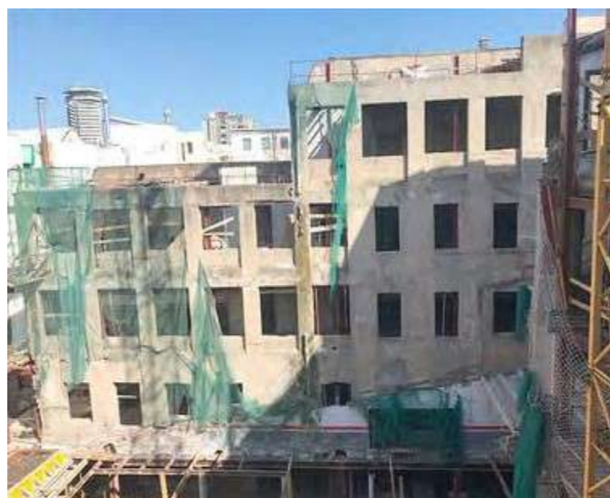
Fig.1-2: Views of the existing conditions of the courtyards façades. © Juli Pérez-Catalá Arquitectura
