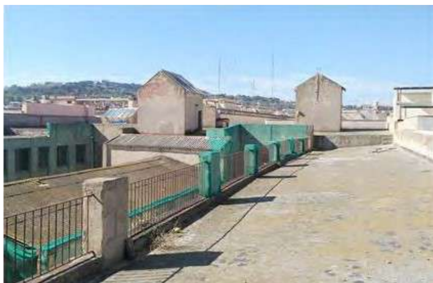
Fig.5-6: Views of the existing conditions of both roof systems. © Juli Pérez-Catalá Arquitectura
