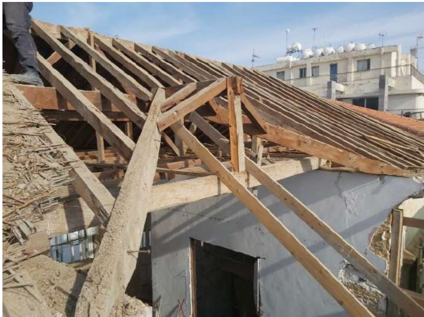
Fig.10: Exterior view of the roof during restoration works. © Simos Drousiotis/A. M. Andronicou Ltd
