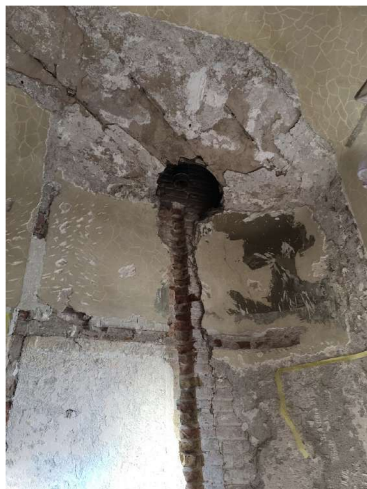
Fig 4. Previous condition of the North corner of the North room main facade. A vertical cut, missing stucco and underlying remains that appeared under layers of paint can be see.
