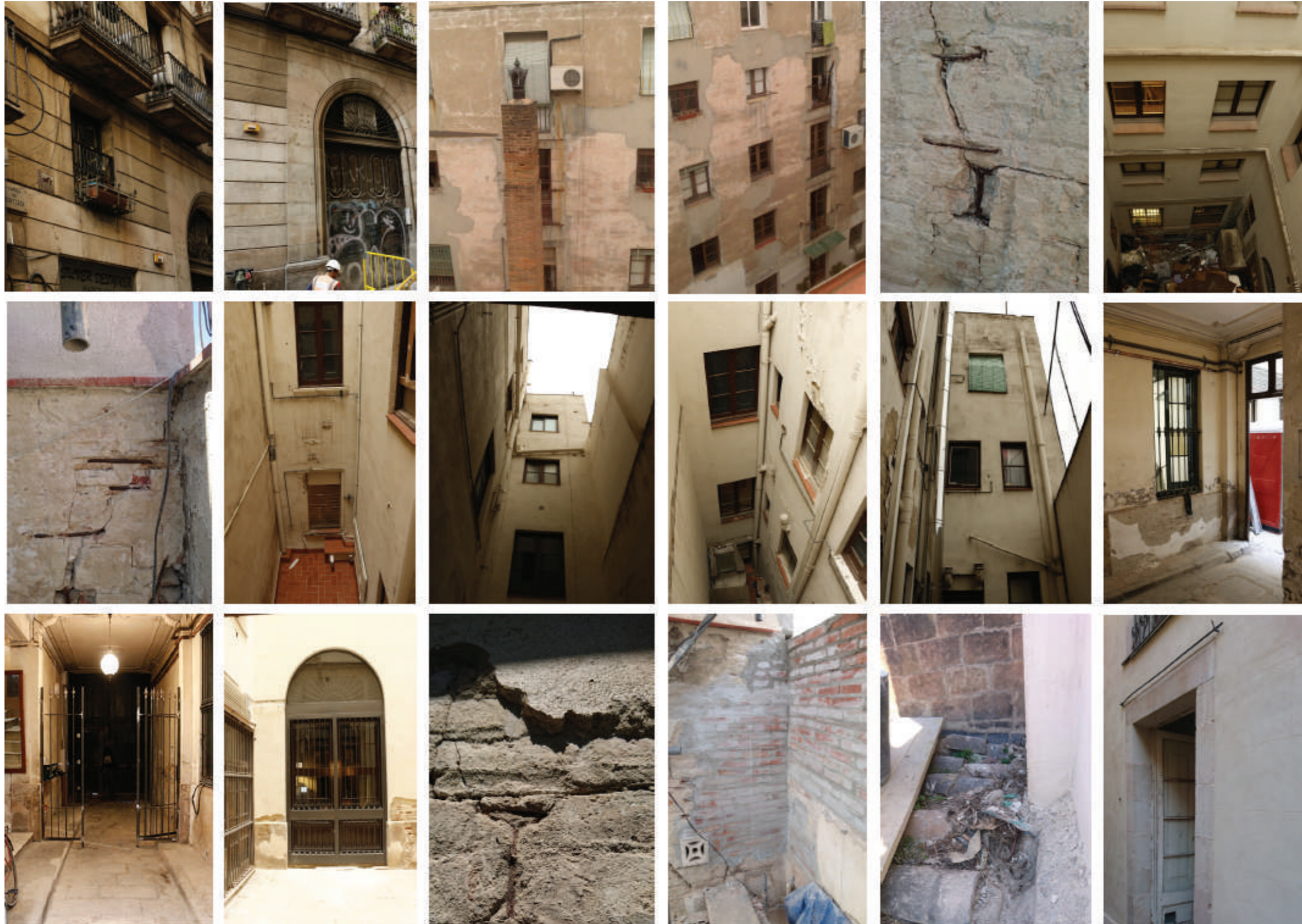
Fig.9: Existing conditions of the building envelopes.
