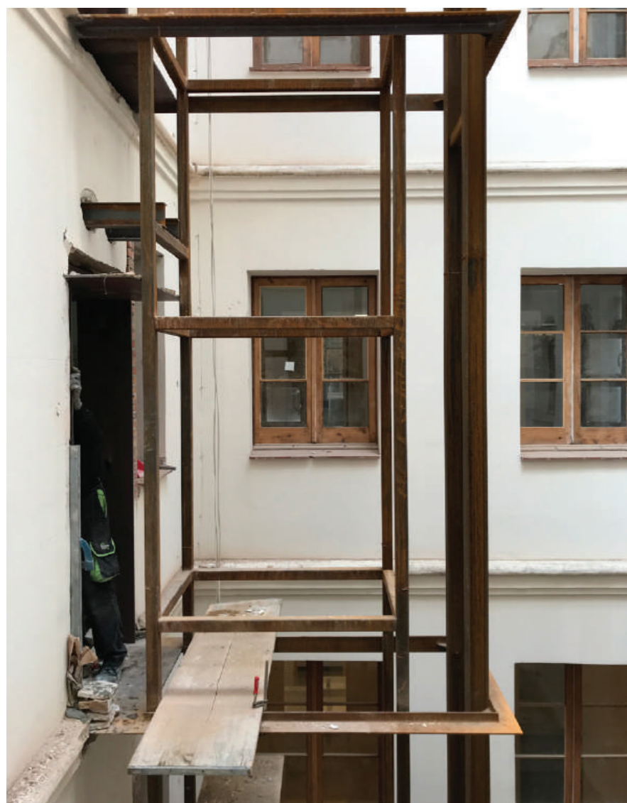
Fig.9: Installation of the elevator's steel frame, and enlargement and reinforcement of the openings to improve accessibility.
