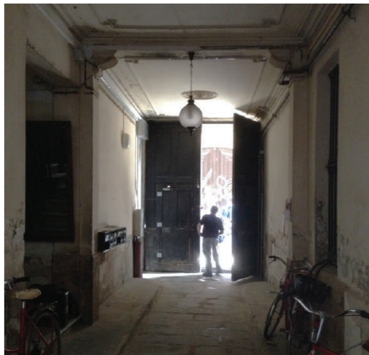
Fig.1: View of the entrance from the inside of the building, before the intervention.
