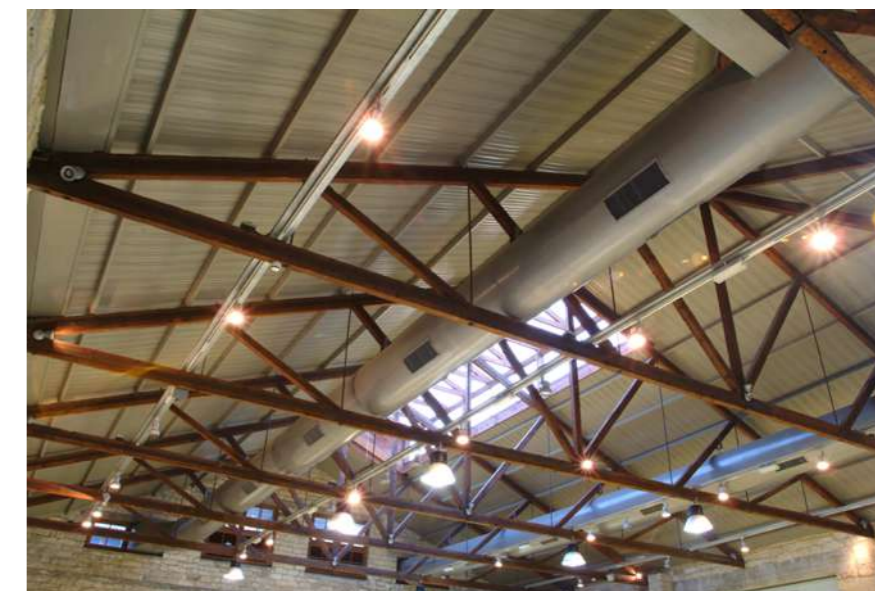
Fig.11: All air-conditioning ducts and light tracks are exposed in the roof truss zone. © Kristian Christou Architects, A. J. Brooks, Architect.
