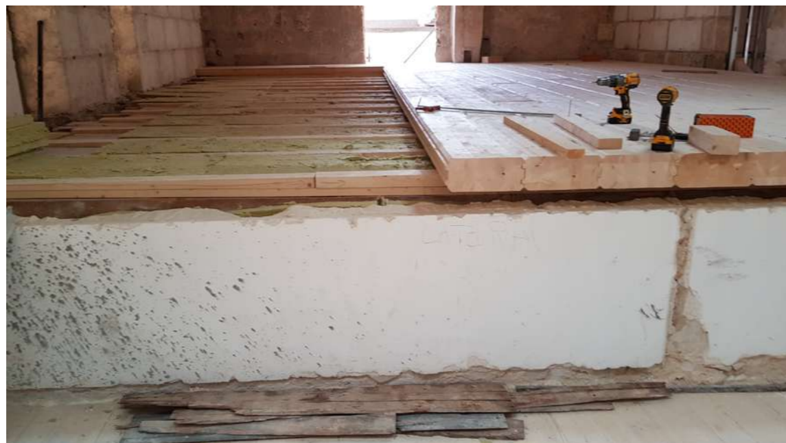
Fig.43: Reinforcement of ancient floor slabs through “tongued and grooved” laminated wood beams, both connected.
