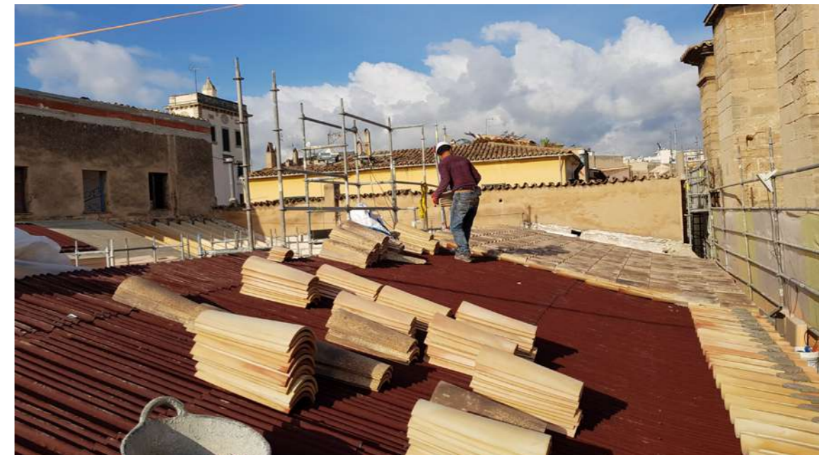
Fig.37: Finishing the roofs with a combination of recovered old tiles and new ones.
