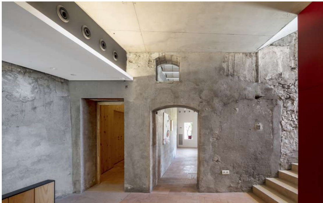
Fig.12: View of a rehabilitated space of transition on the inside of the building.
