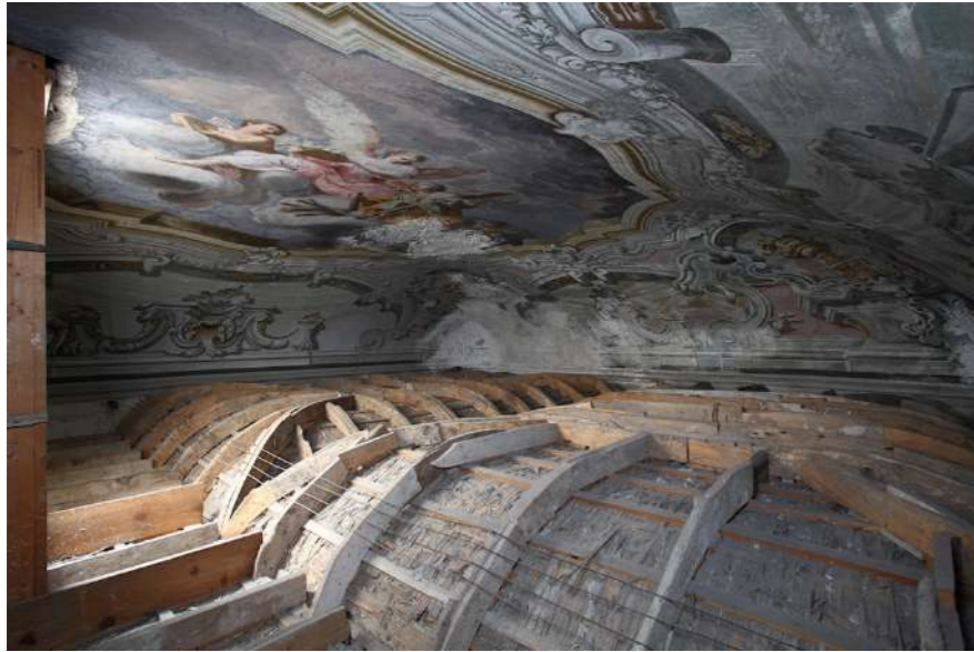
Fig.22a-b: Decorated thin sheet bricks vaults hidden by other wooden ceilings, before restoration, restoring frescoes in the reception rooms of the palace. © Project Designers & Francesco Renda.
