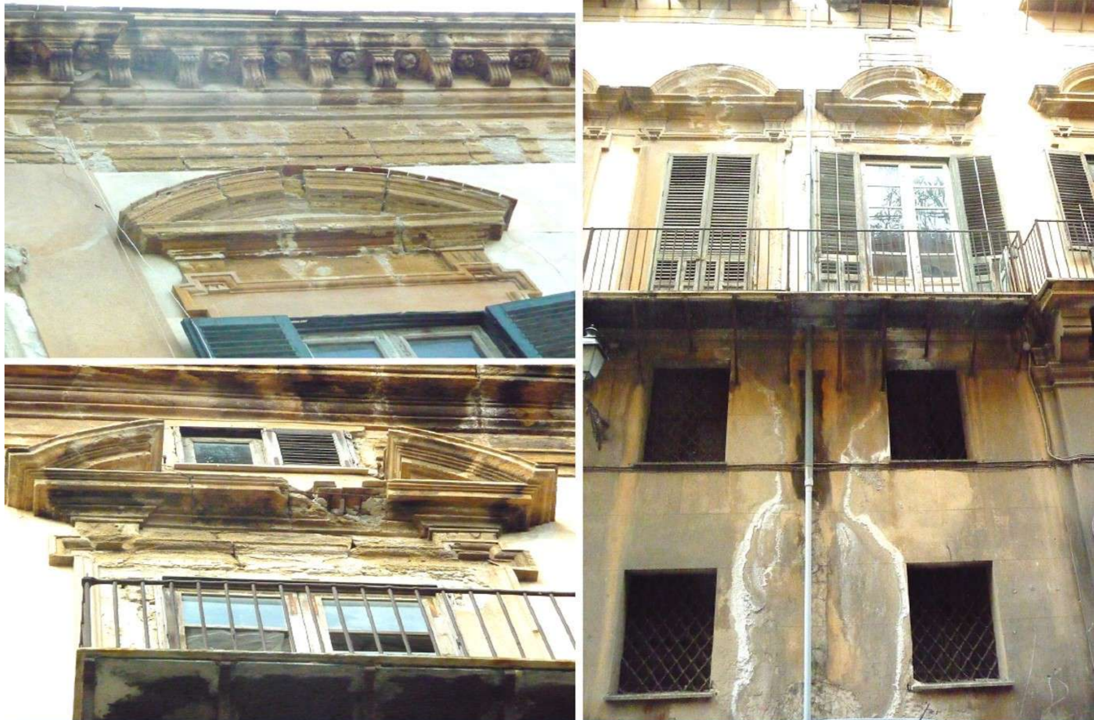
Fig.11: Façade damages of stone and stucco or plasters. © Project Designers
