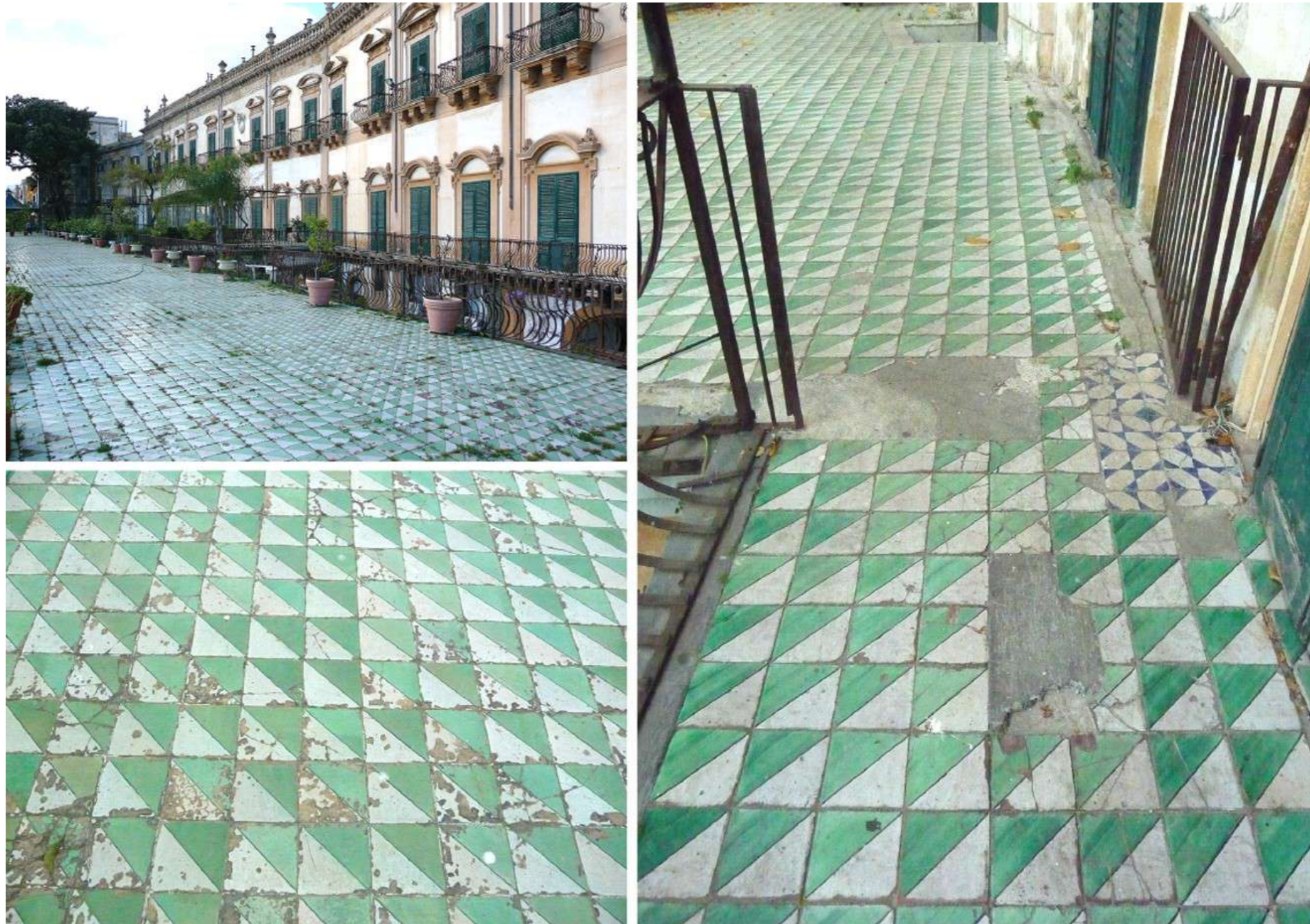
Fig.13: Decay of the indoor and outdoor majolica paving. © Project Designers
