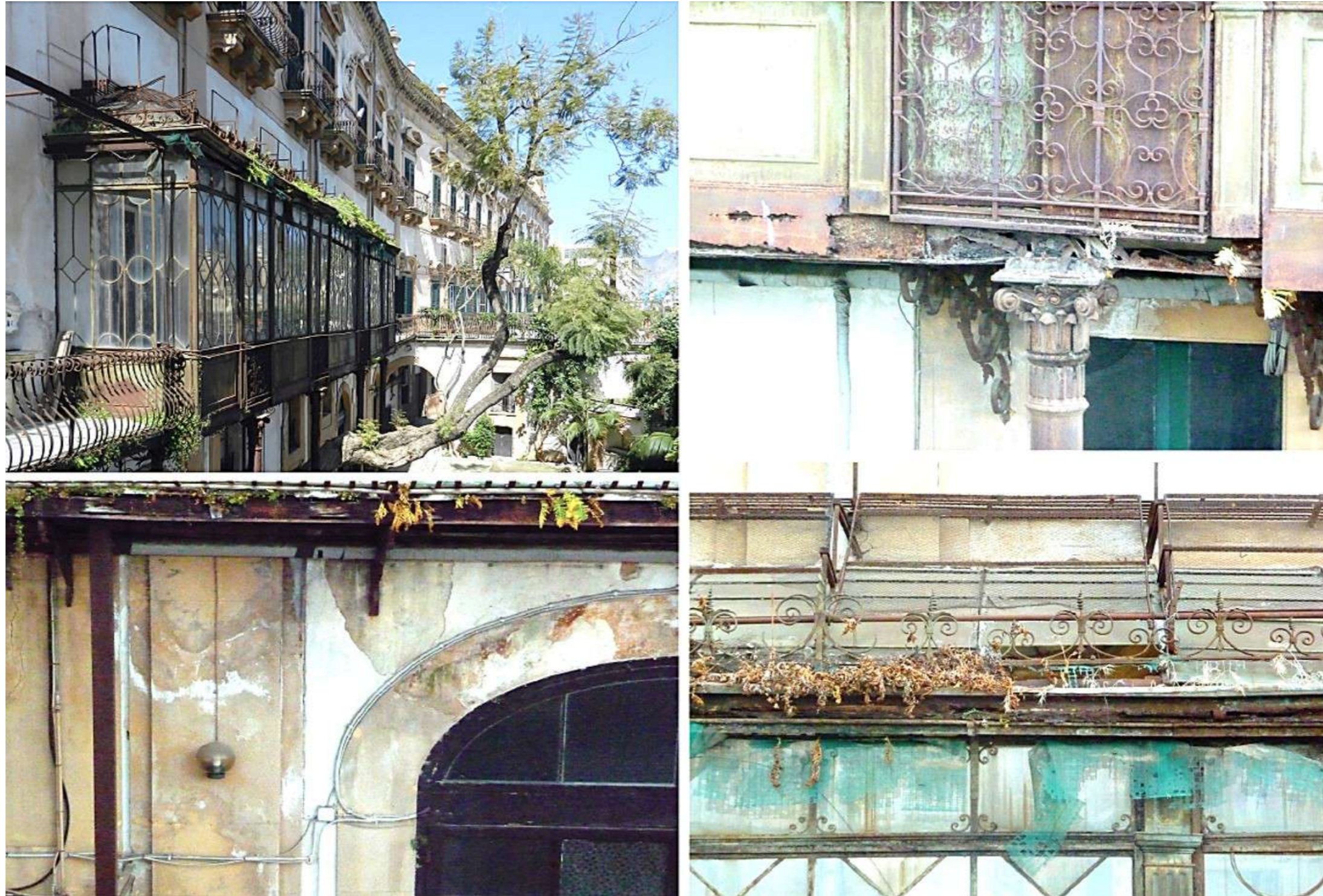
Fig.12: Decay of metal structures and elements in the internal façade overlooking the internal courtyard. © Project Designers
