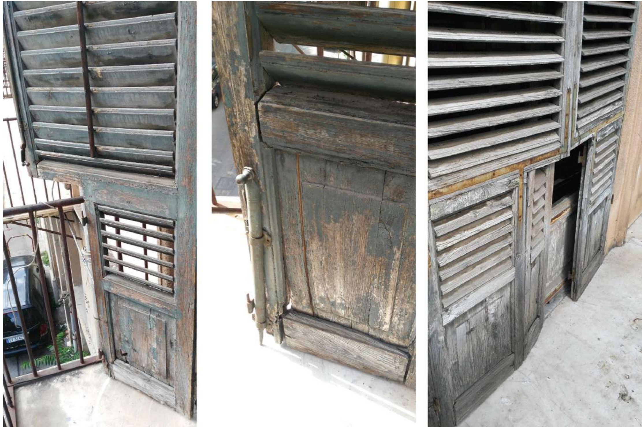
Fig.14: Deterioration of wooden window frames. © Project Designers
