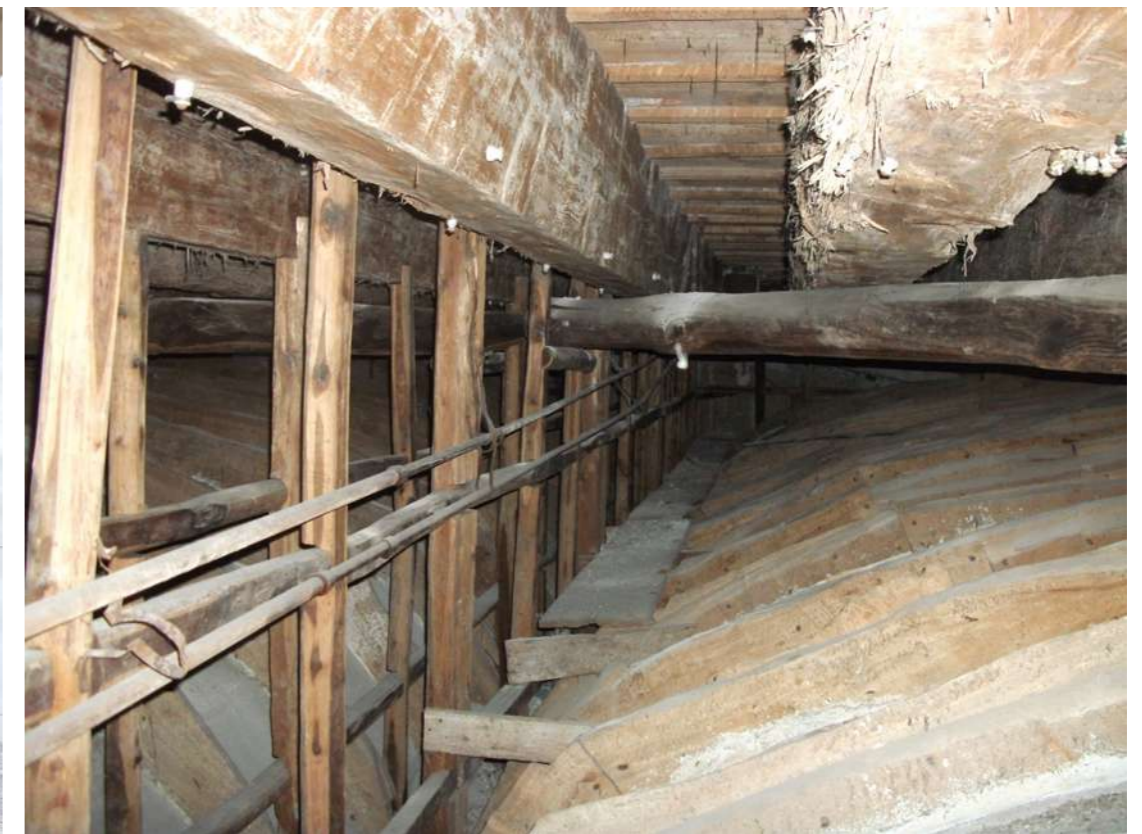
Fig.7: Butera palace, details of a wooden floor and the vaulted ceiling, before the restorations. © Project Designers
