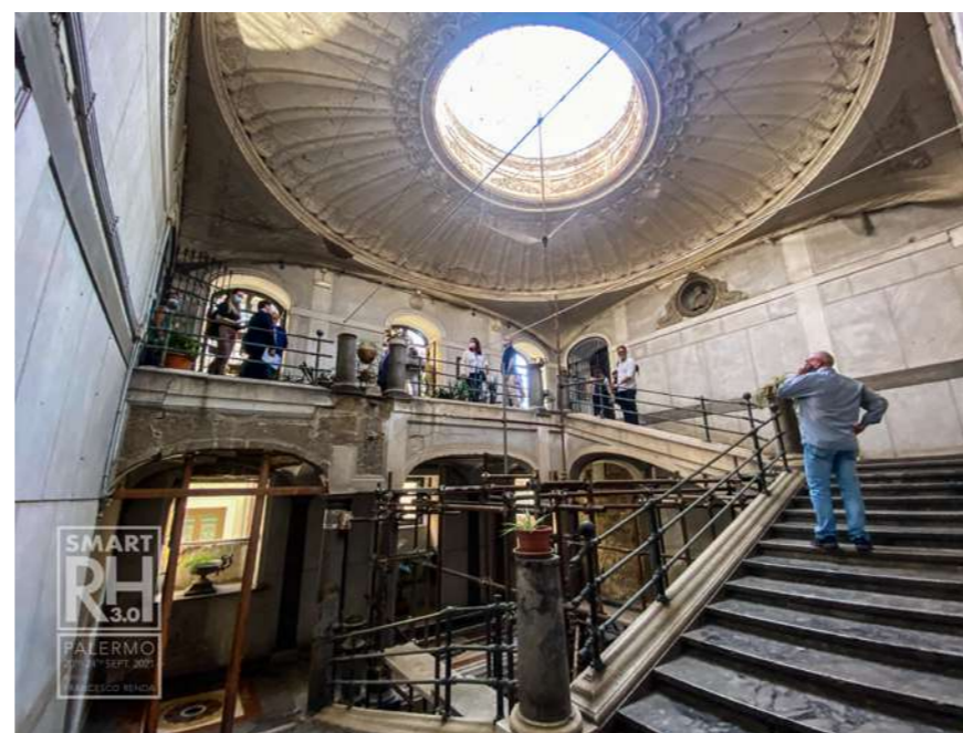
Fig.27: The monumental staircase of the Cattolica-Briuccia palace, one of the building that constitute the luxury hotel, with its deterioration and instability decay, awaiting restoration during the Staff Training Course (C6) of the EU Smart Rehabilitation 3.0 project, Palermo September 2021. ©Francesco Renda
