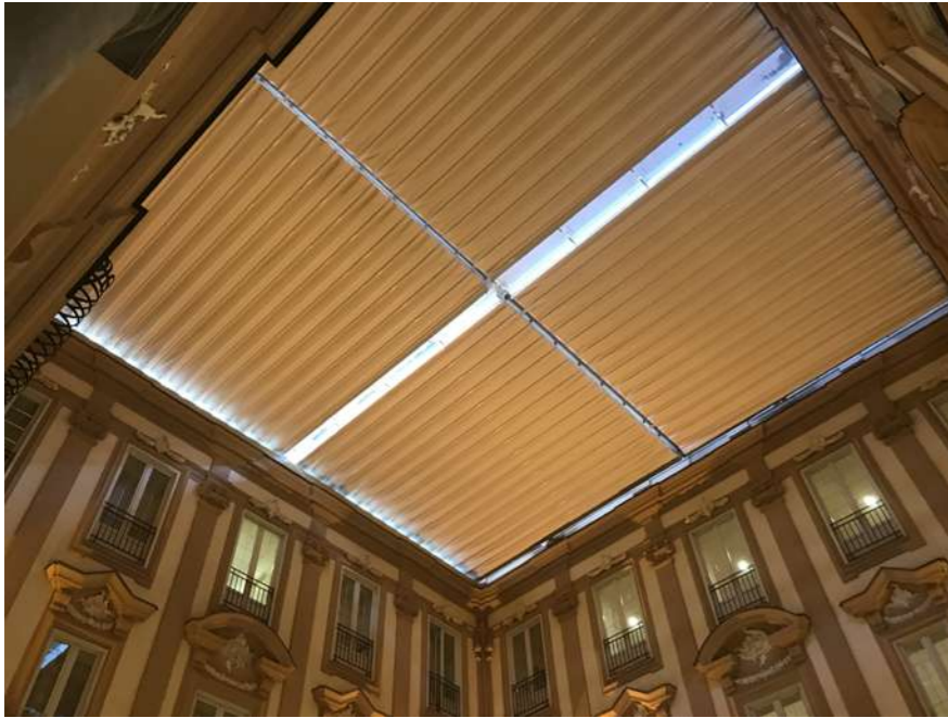
Fig.44: The same skylight-curtain that closes the ancient four-sided portico of the former convent from above, when it is closed. © Tiziana Campisi
