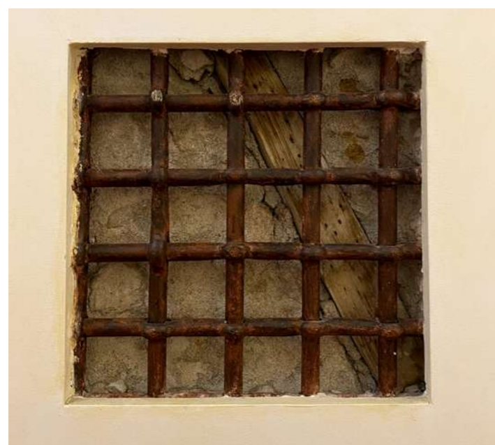
Fig.24: All the restoration interventions were based by the respect for the discovery of surviving elements, highlighted and enhanced, without depressing or replacing them, in a system of recognizability. ©Luisa Lombardo
