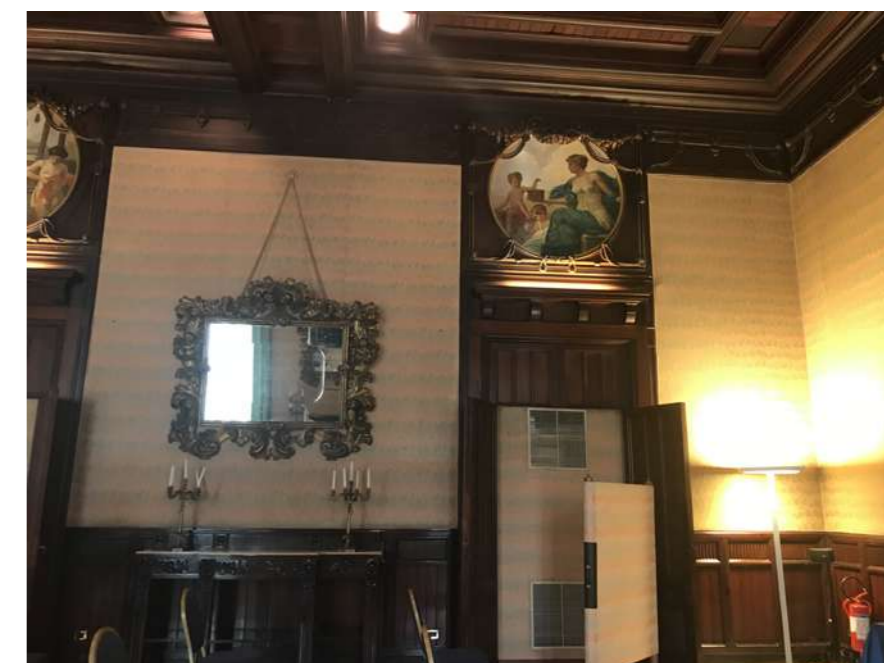
Fig.30: Liberty interior spaces of the former Cassa di Risparmio bank converted into a conference room; the large doors presenting a big thickness host the air conditioning and heating systems. ©Tiziana Campisi
