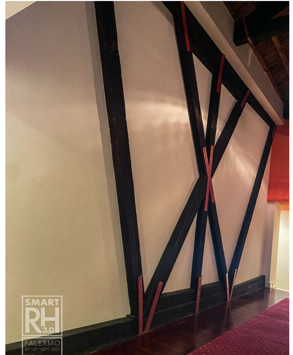
Fig.39: Reinforcement and bracing system of of an interior wall using a wooden frame. ©Francesco Renda
