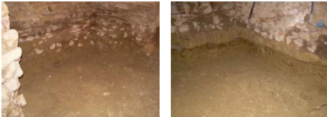
Fig.3-4: State of the foundation masonry before the consolidation intervention.
